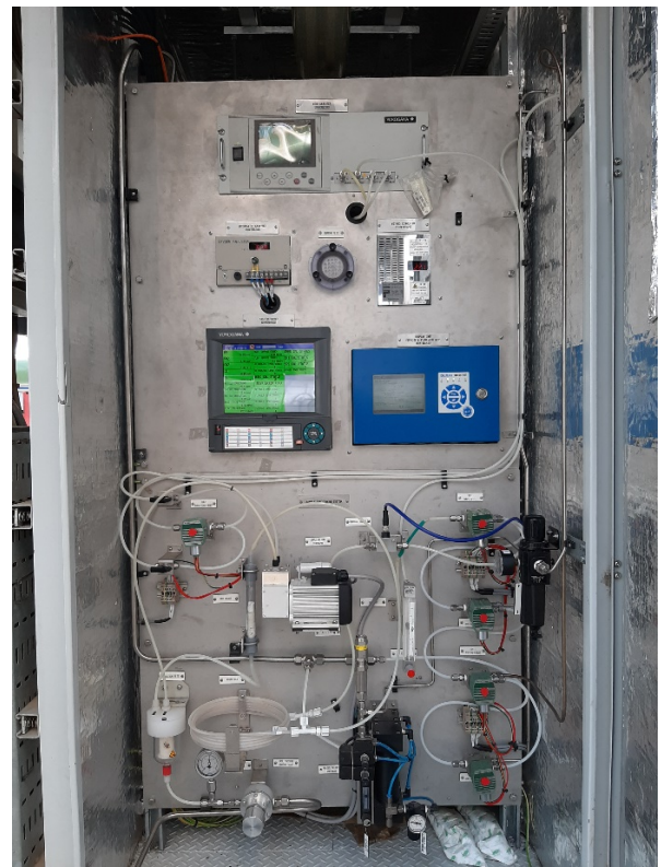
Analyzer Inside CEMS Cabinet (Identical for the 2 units)
