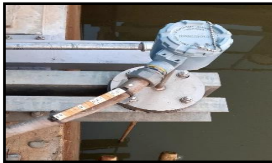
Figure 3.2 Temperature Sensor Location at Central Monitoring Basin
