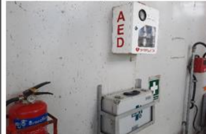
AED device and first aid box are ready to use in case of emergency
