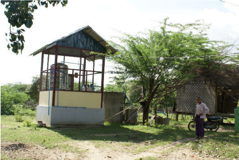
UV/UF water treatment system
