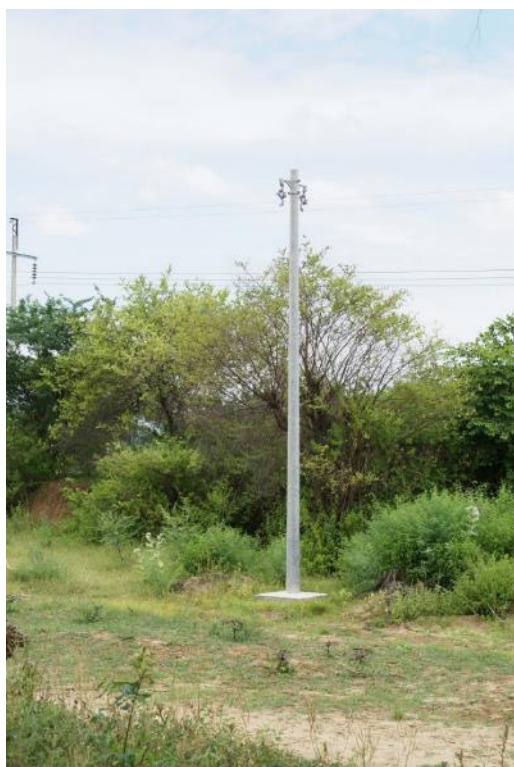
Photo 40: Power Pole along the river water supply pipeline
