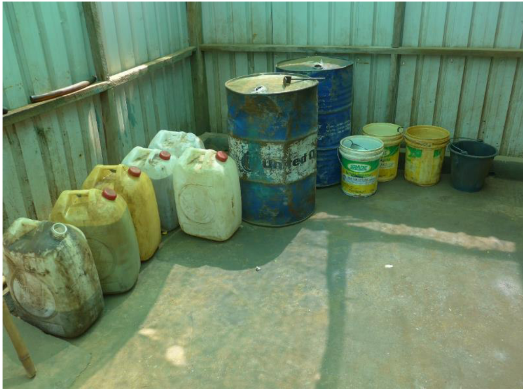
Photo 13: Several drainage holes in bund wall around diesel tank in SDCI area (most are obscured by the drums)
