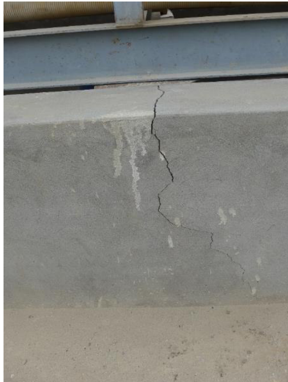
Photo 11: Cracks in bund wall around diesel tank at Concrete Batching Plant
