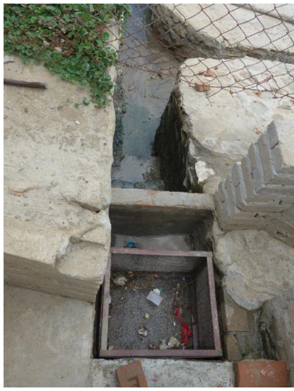
Photo 8: Screen on kitchen wastewater discharge at JEM camp
