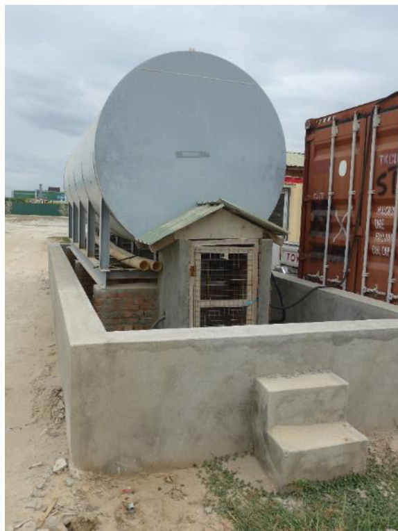
Photo 12: Drainage pipe from bunded area (bottom left of photo) had an open valve
