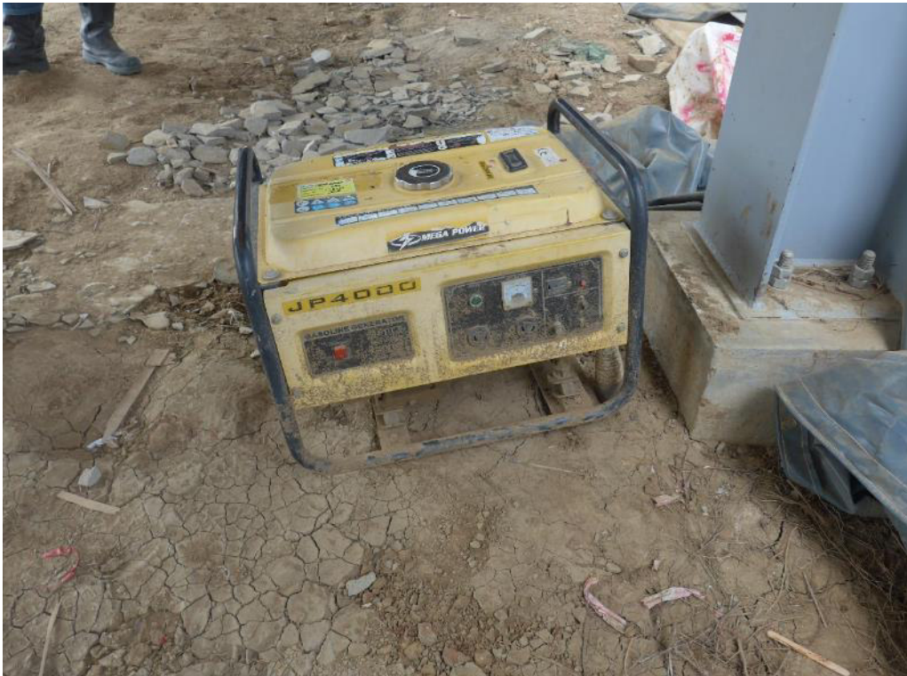
Photo 15: Portable generator without a drip tray
