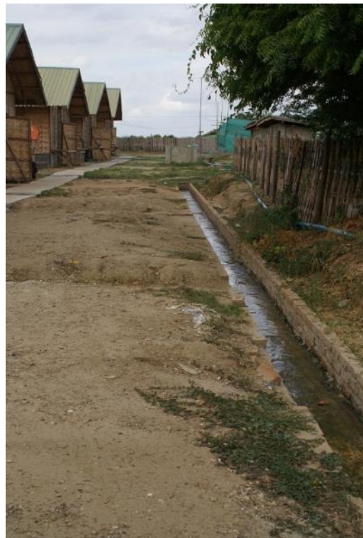
Photo 28: New drainage system at Min Dhama camp
