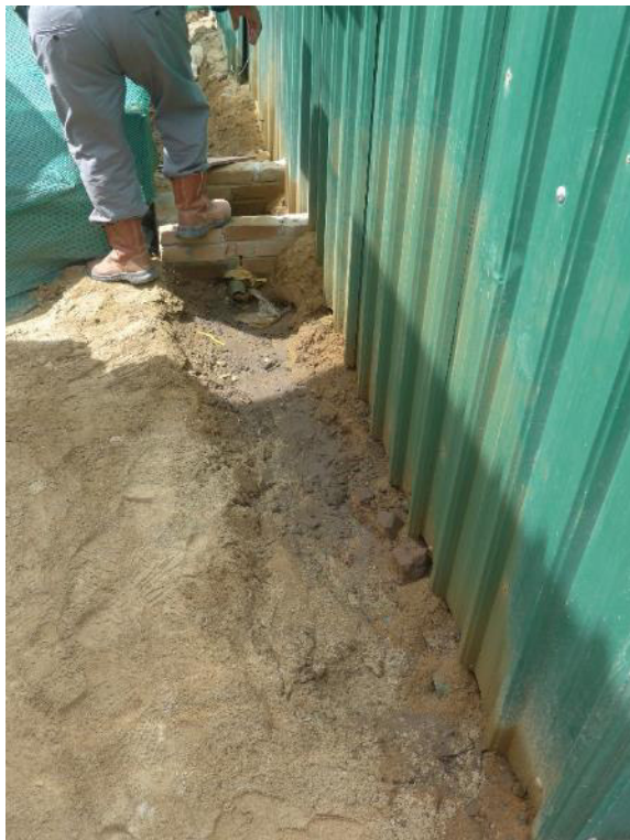
Photo 14: Soil contamination outside diesel tank in SDCI area
