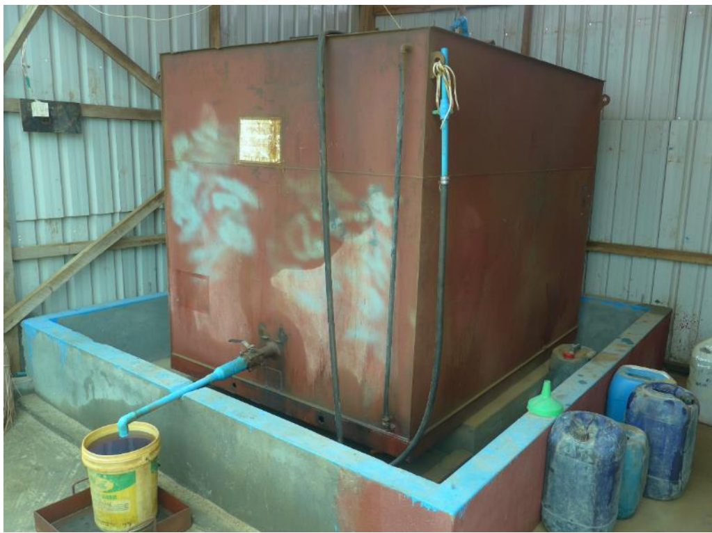
Photo 10: Bund appears to have less than 110% of the tank capacity
