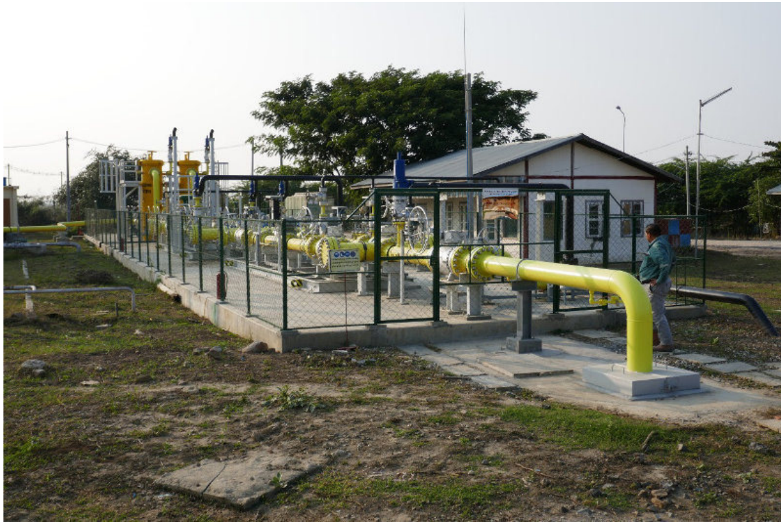
Photo 1: MOGE gas receiving station
