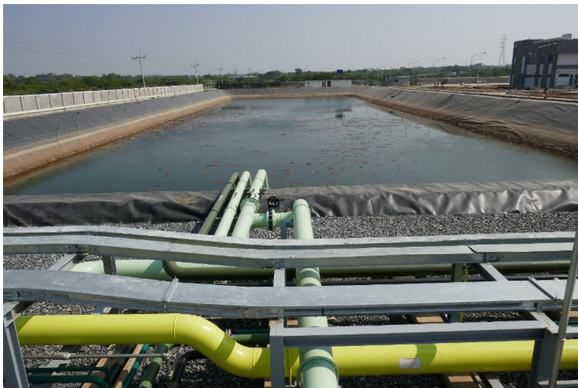
Photo 13: River water storage reservoir
