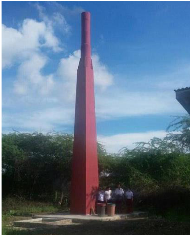
Photo 29: Medical waste incinerator at Myingyan Hospital
