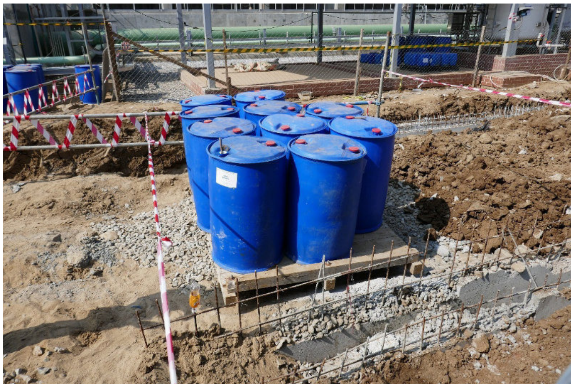
Photo 22: Sodium hypochlorite tanks with no secondary containment
