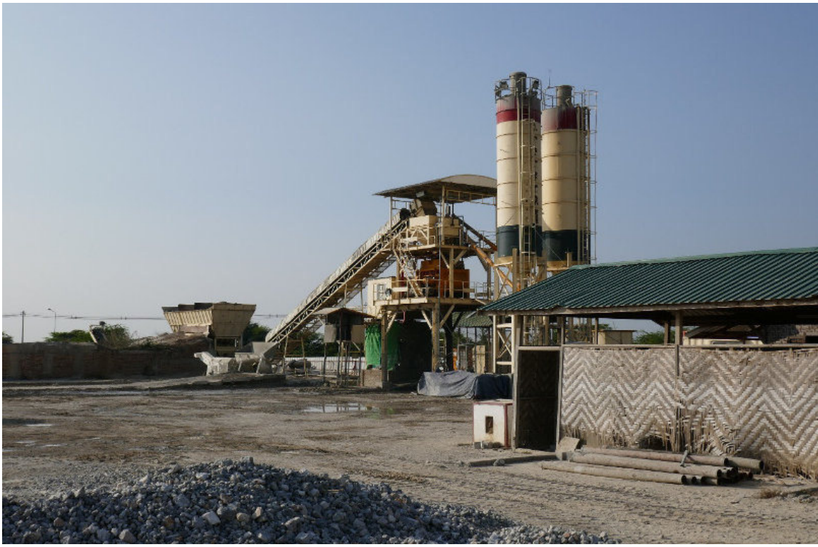
Photo 9: Enclosed conveyor at concrete batching plant
