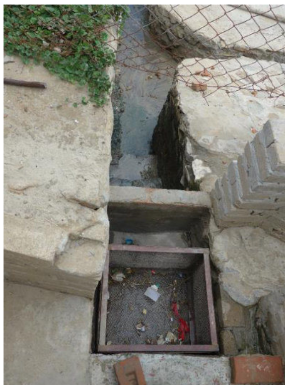
Photo 18: Screen on kitchen wastewater discharge at JEM camp
