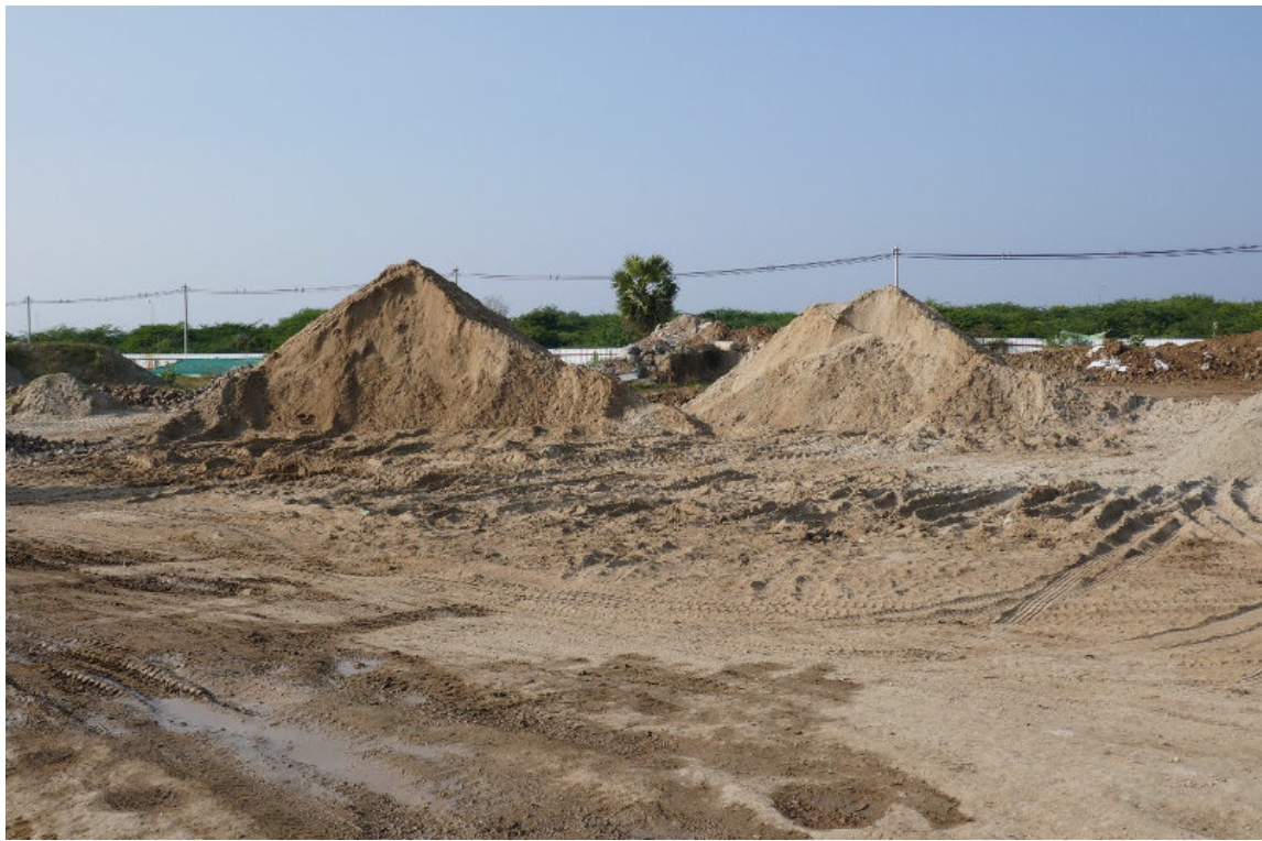
Photo 10: Soil stockpiles exceeding 2 m high
