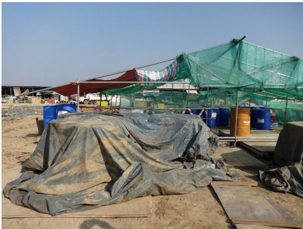
Photo 24: Storage of chemicals and oil without secondary containment
