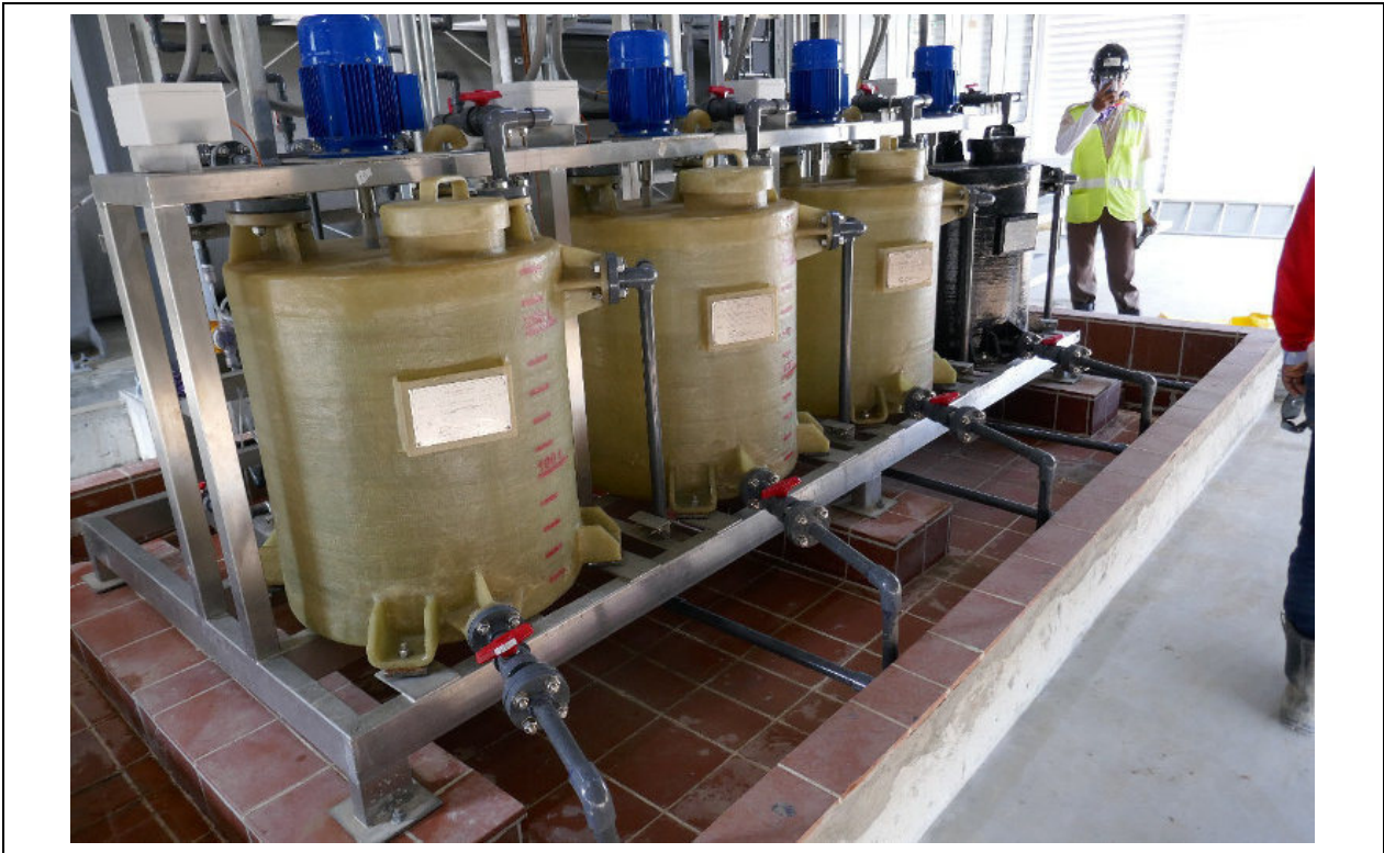
Photo 19: Sewage treatment plant
