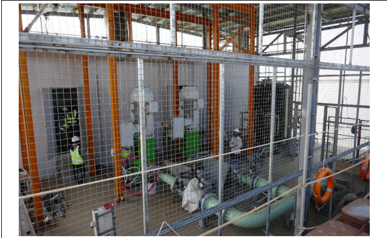
Photo 12: River water intake pumps
