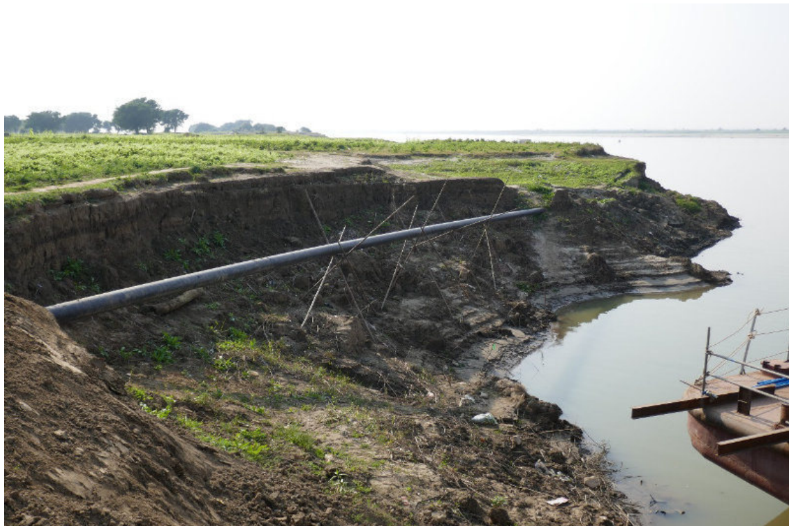
Photo 3: Wastewater pipeline exposed by river bank erosion
