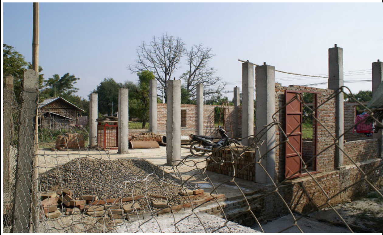
Photo 43: Foundation for the farmer's new house and shop along the river water supply pipeline
