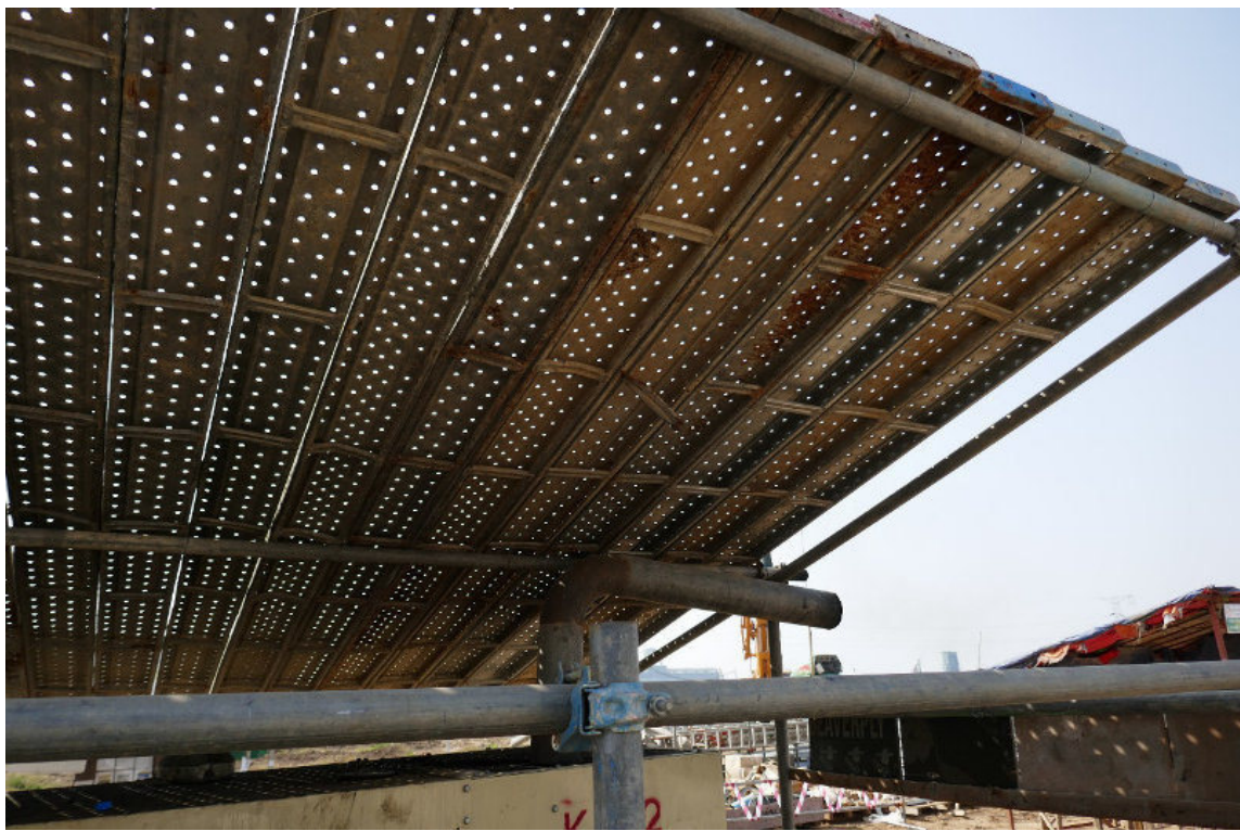
Photo 26: Non-watertight roof over a diesel generator
