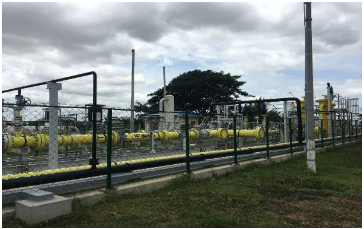
Photo 17: MOGE gas receiving station
