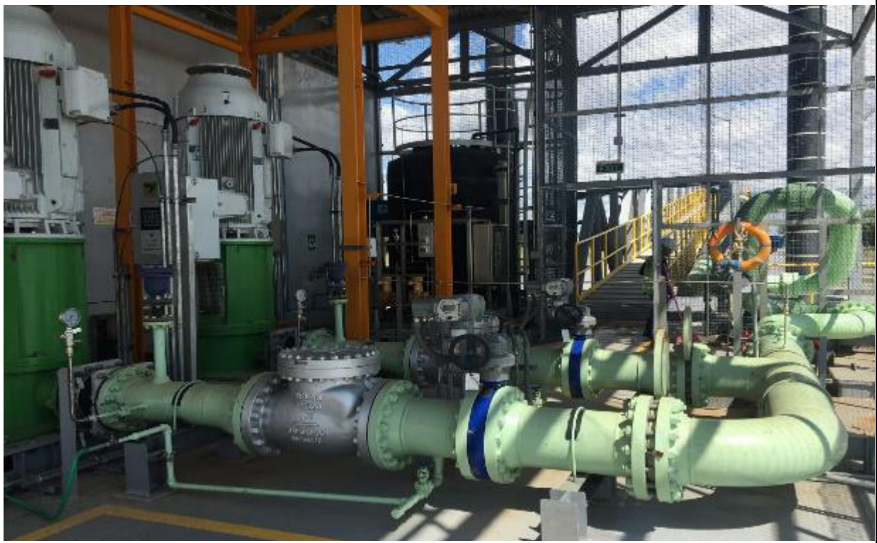
Photo 20: River water supply pumps
