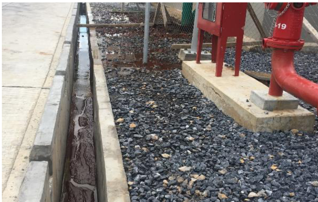
Photo 6: The water sludge mixture overflowed onto the gravel layer surrounding the recycle water tank and an adjacent internal drain
