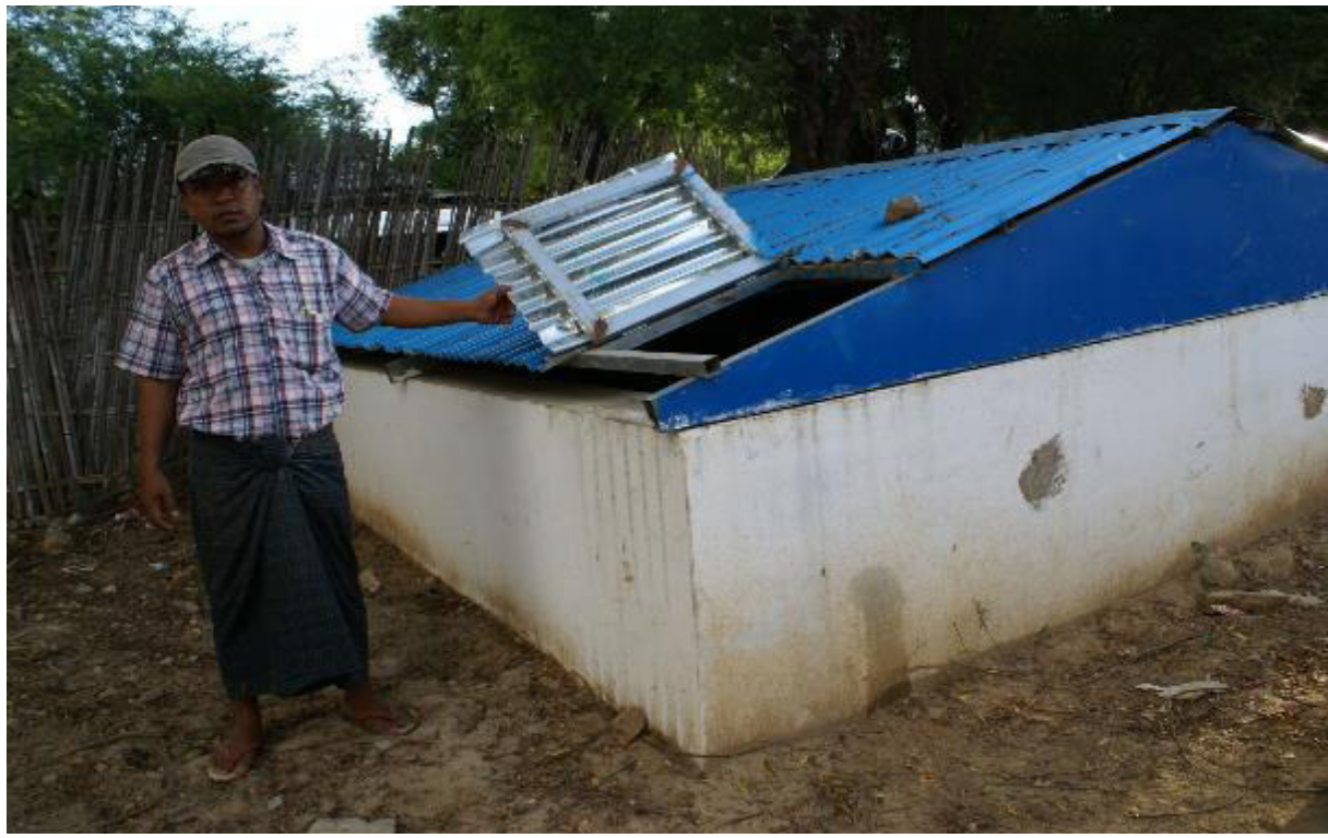
Photo 33: Nyaung Kan Village: 500-gallon underground tank for fire protection, a Sembcorp/PCo CDP Project
