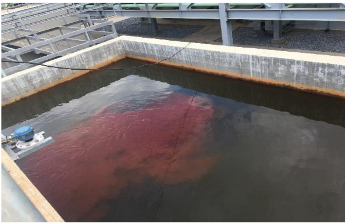
Photo 5: A faulty agitator in the sludge thickener tank resulted in an overflow of water sludge mixture into the recycle water tank.
