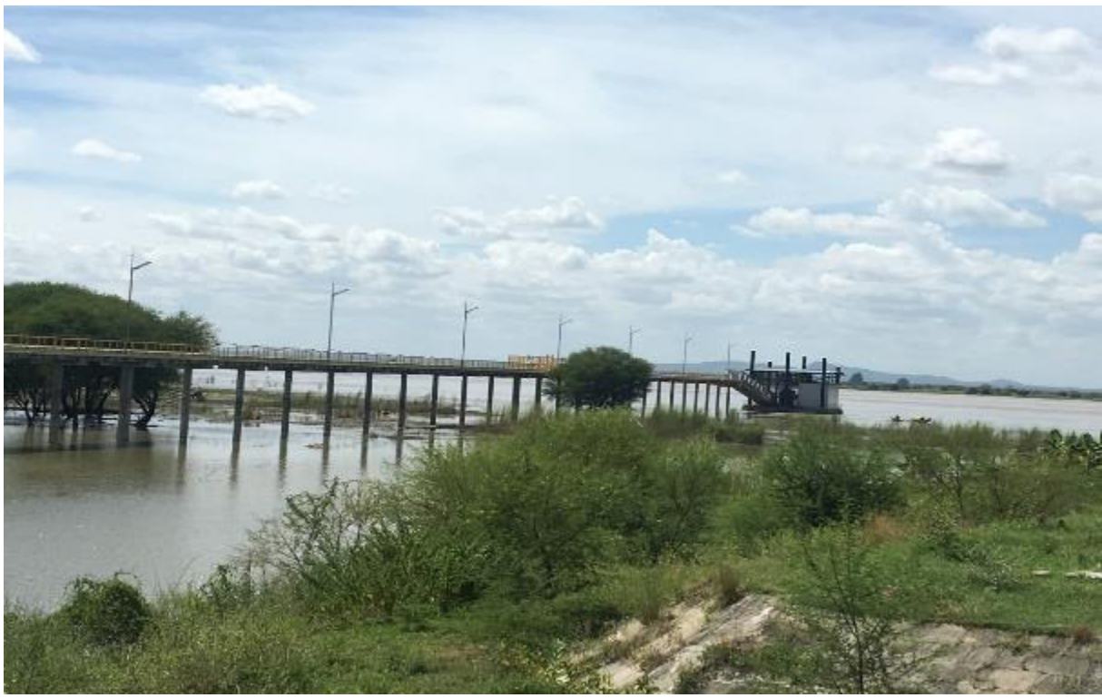
Photo 19: Overview of the river water supply pipeline and pumping station
