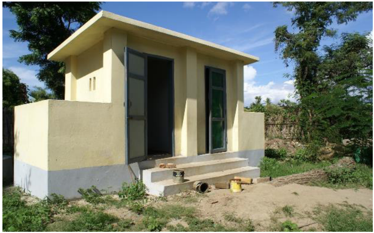
Photo 27: Tha Pyay Thar Village: New toilets built at the primary school, a Sembcorp/PCo CDP Project
