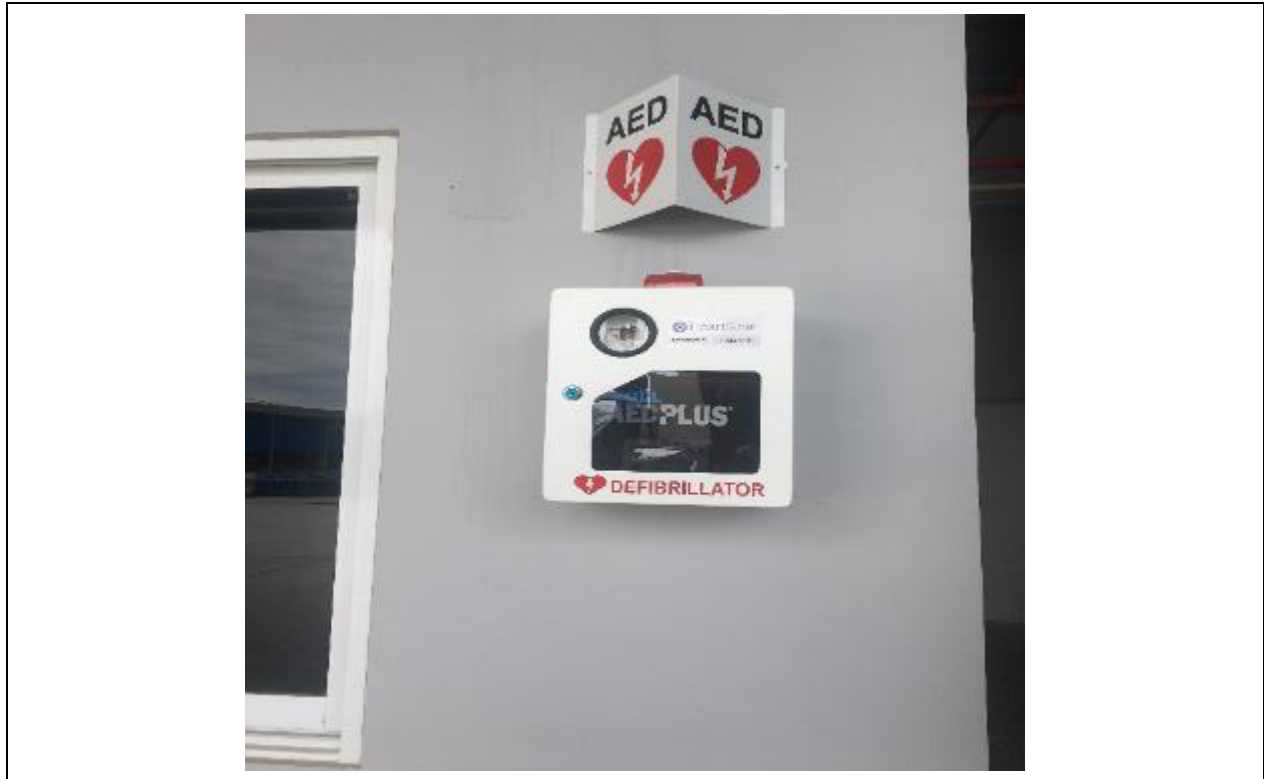
Photo 11: The site has installed four (4) automated external defibrillators (AEDs) onsite.
