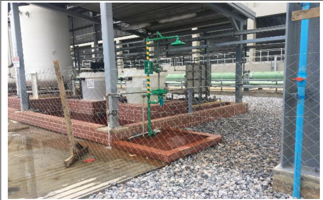
Photo 7: The excess sludge water mixture overflowed into adjacent chemical feed storage areas (up to one inch of water on the floor).
