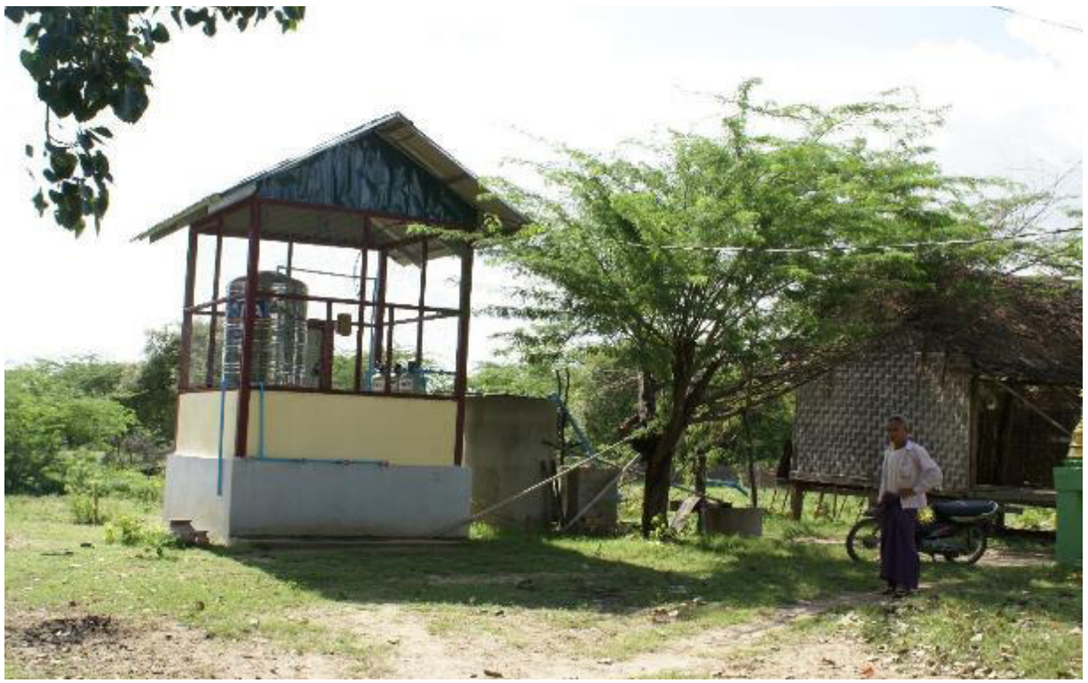
Photo 25: Tha Pyay Thar Village: Solar-powered water treatment facility, a Sembcorp/PCo CDP Project
