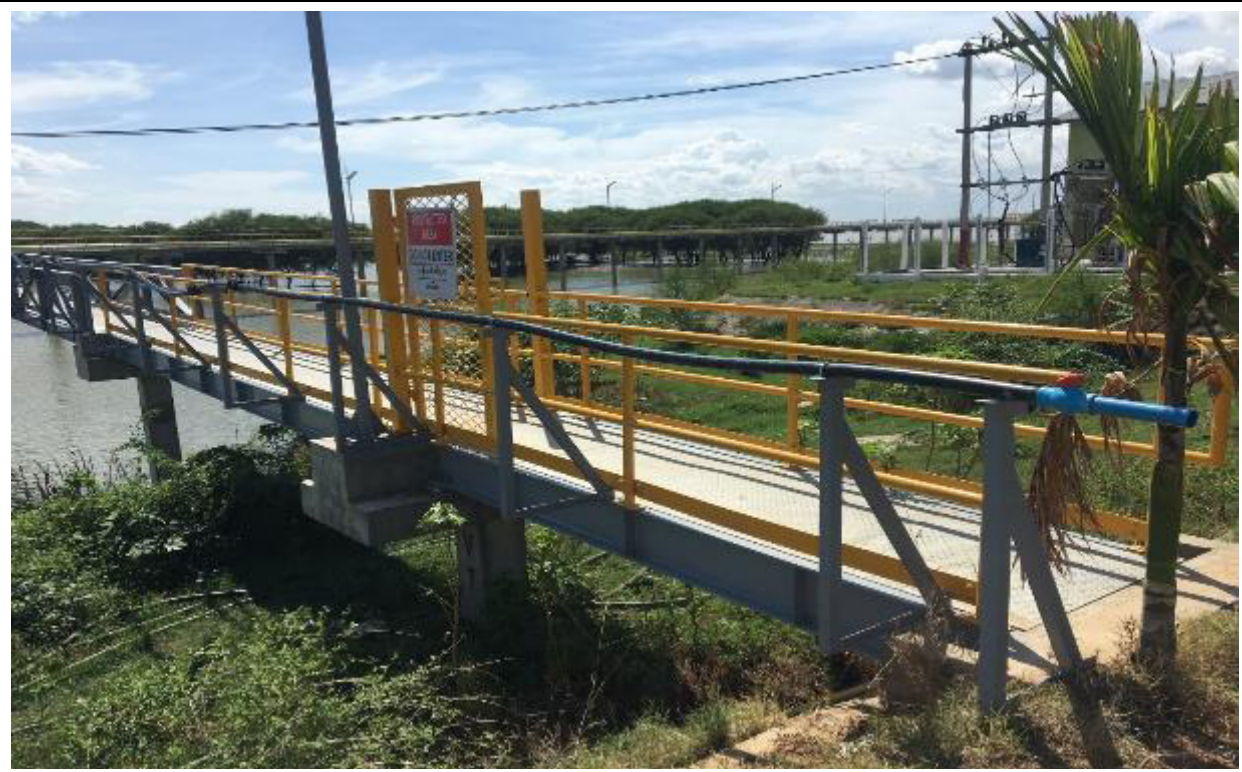
Photo 18: Secured entrance leading to the river water supply pumping station
