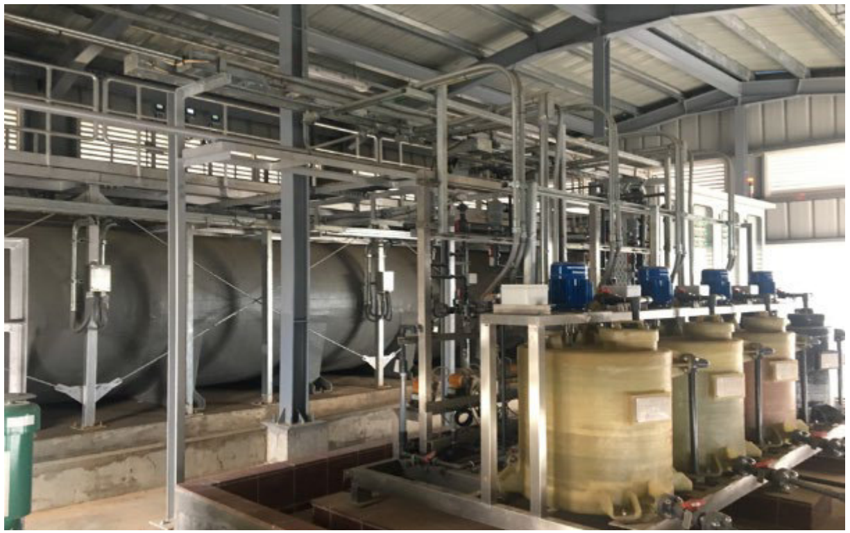
Photo 9: Sanitary wastewater treatment plant. All sanitary wastewater from the site is routed to the plant from April 2018 onwards
