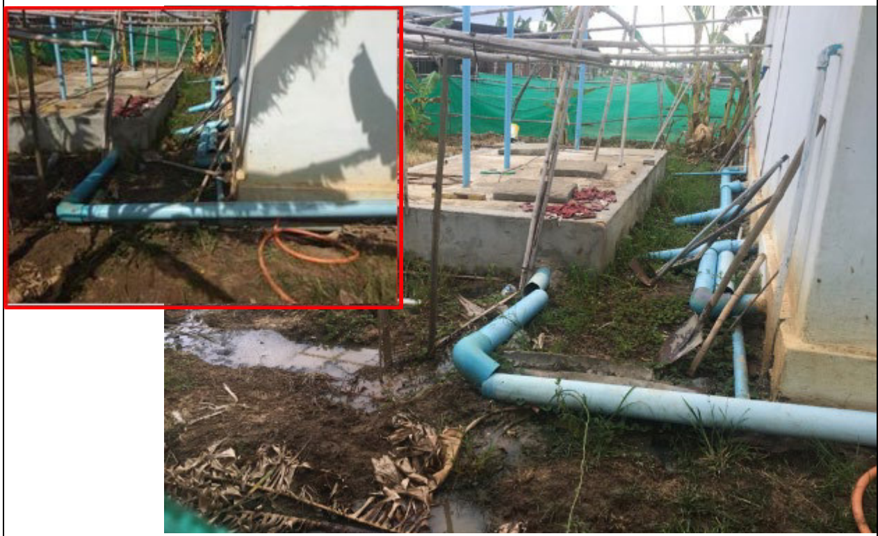
Photo 13: The toilet at the JEM Office had a broken pipe leading from the sink into the cess pit. Inset: The pipe was replaced a day later.
