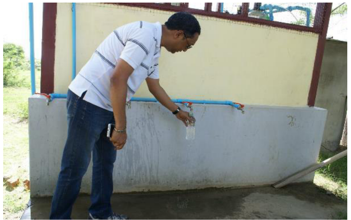
Photo 26: Tha Pyay Thar Village: Potable water produced from the solar-powered water treatment facility, a Sembcorp/PCo CDP Project
