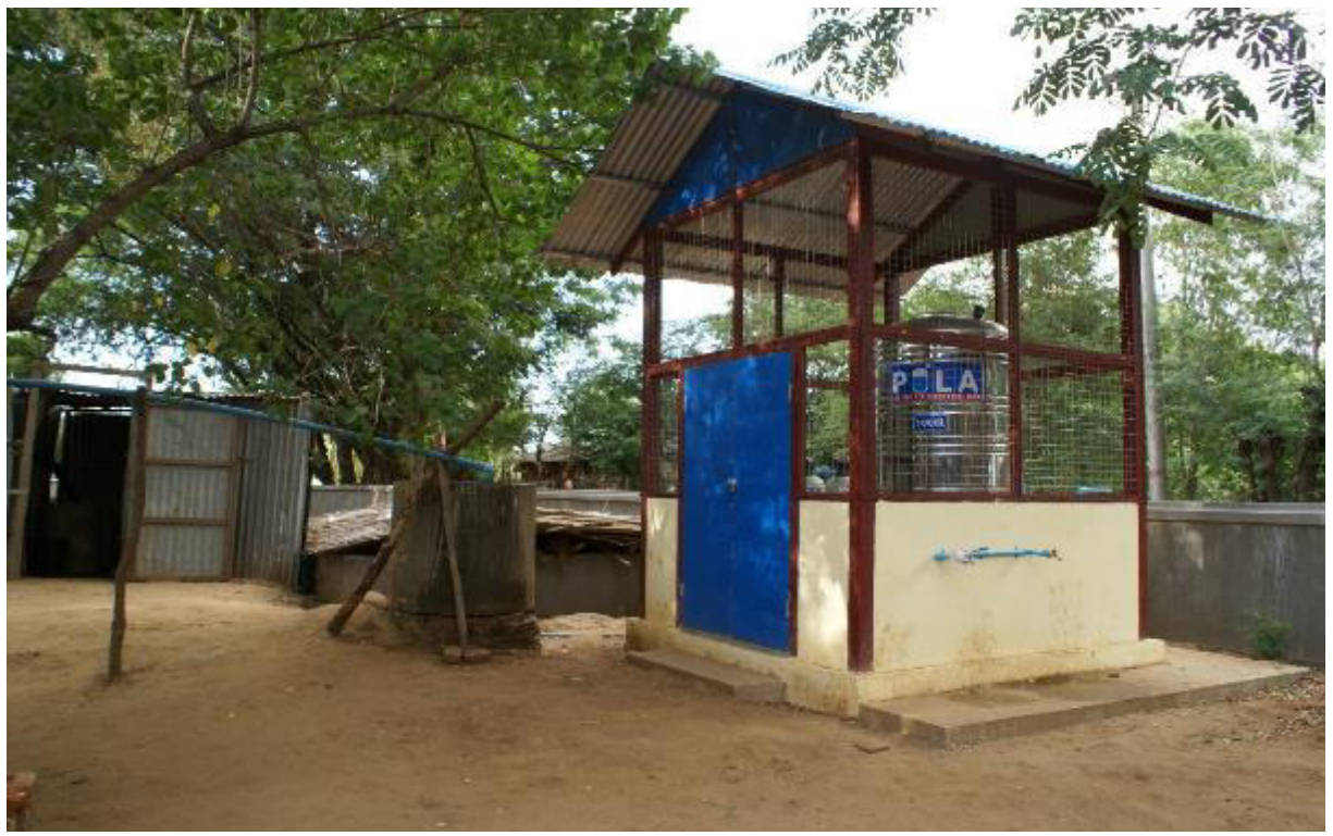
Photo 31: Nyaung Kan Village: Solar-powered water treatment facility, a Sembcorp/PCo CDP Project
