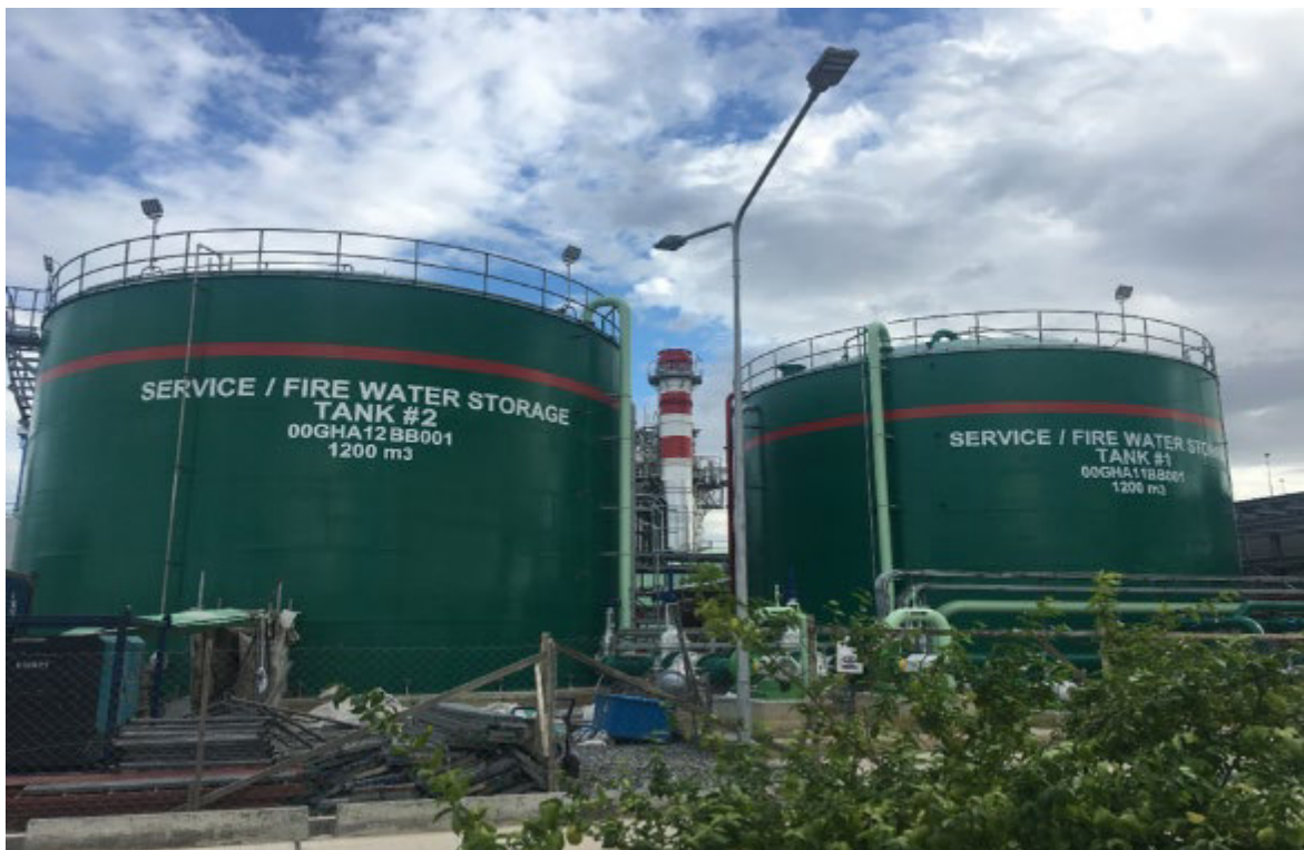
Photo 10: Two (2) fire water storage tanks of 1200 m 3 capacity each
