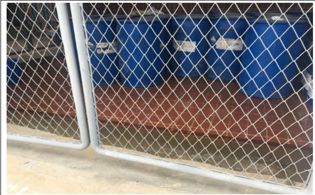
Photo 8: Insufficient containment at the chemical store (for water treatment chemicals) based on the volume of chemicals stored. Floor was inundated with approximately 1 inch of water.
