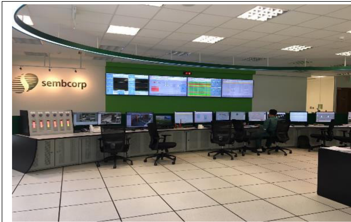
Photo 12: Plant Control Room with Continuous Operations Monitoring System within the main administration building
