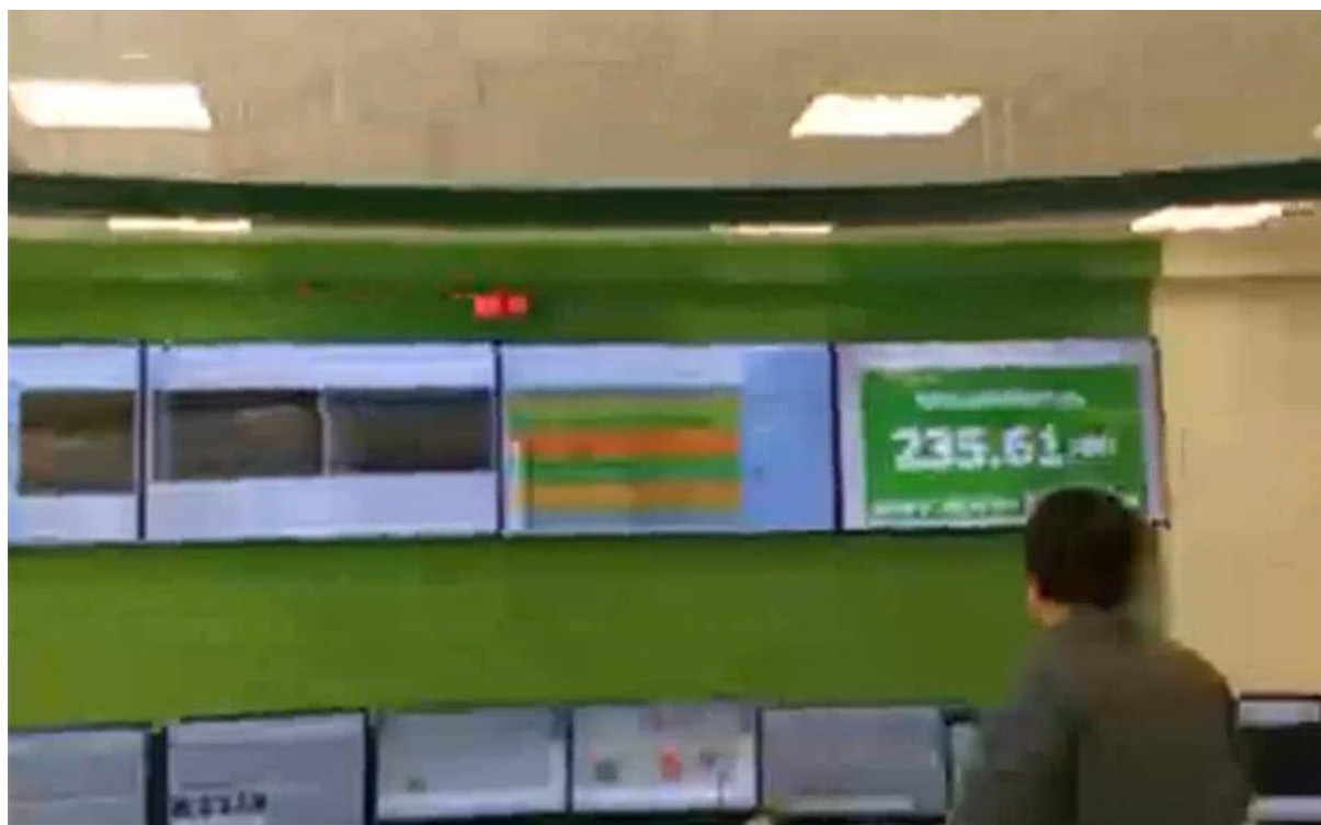
Photo 4: Plant Control Room with Continuous Operations Monitoring System within the main administration building (Photo taken from live video during January 2023 Site Visit)
