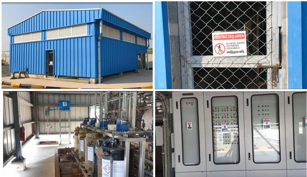
Photo 30: Internal Sewerage Treatment Plant (Photos taken from video shared during January 2023 Site Visit)
