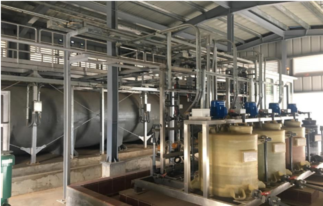
Photo 17: Sanitary wastewater treatment plant (December 2019 Site Visit)
