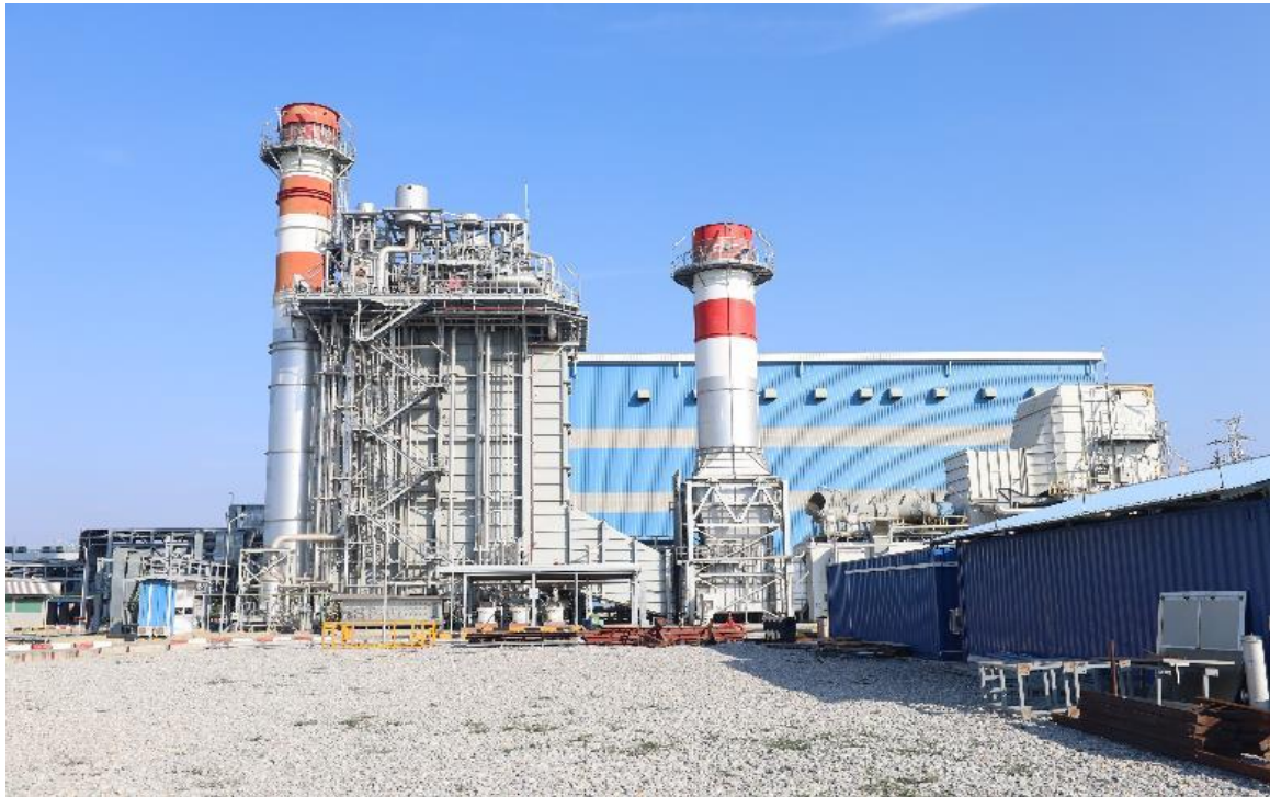
Photo 3: Myingyan CCGT Unit 1 (Photo provided during January 2025 Site Visit)
