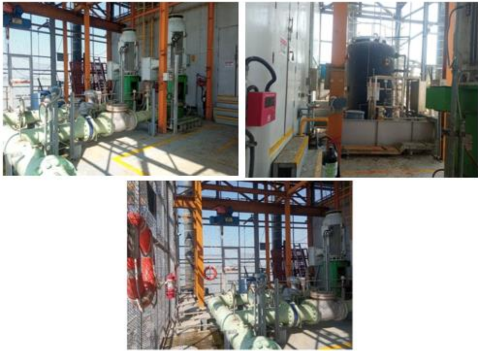
Photo 9: River water intake pumps (Photos provided for January 2024 Site Visit)
