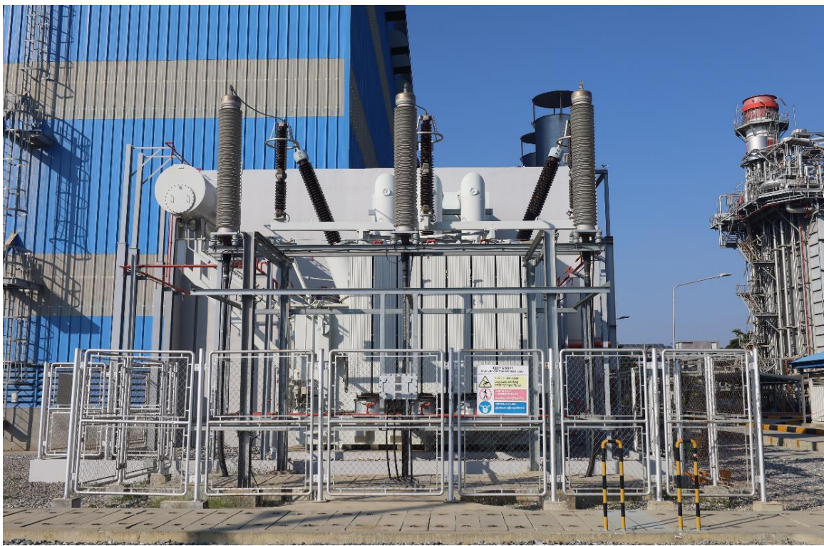
Photo 6: Station Transformer next to Unit 2 (Photo provided during January 2025 Site Visit)
