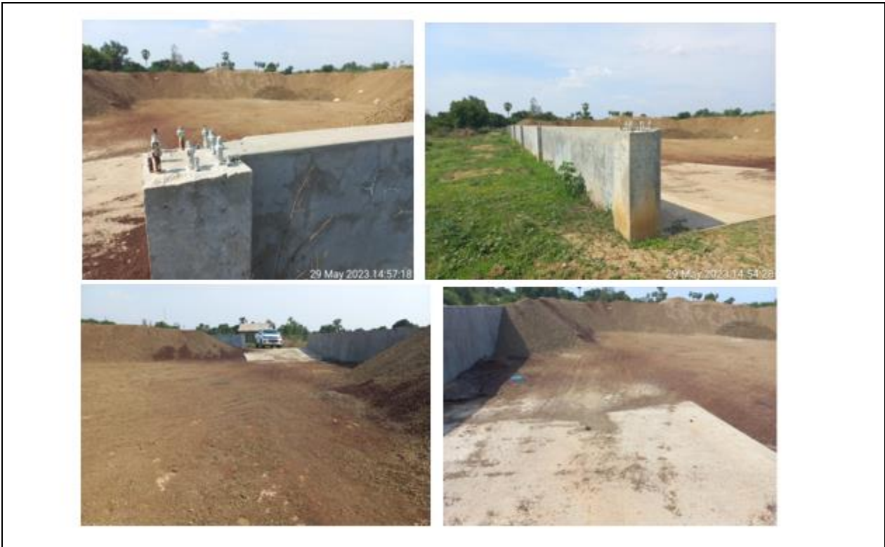
Photo 34: Off-site sludge storage facility owned and operated by OK Service for sludge from the water treatment plant (Photo provided for January 2024 Site Visit)
