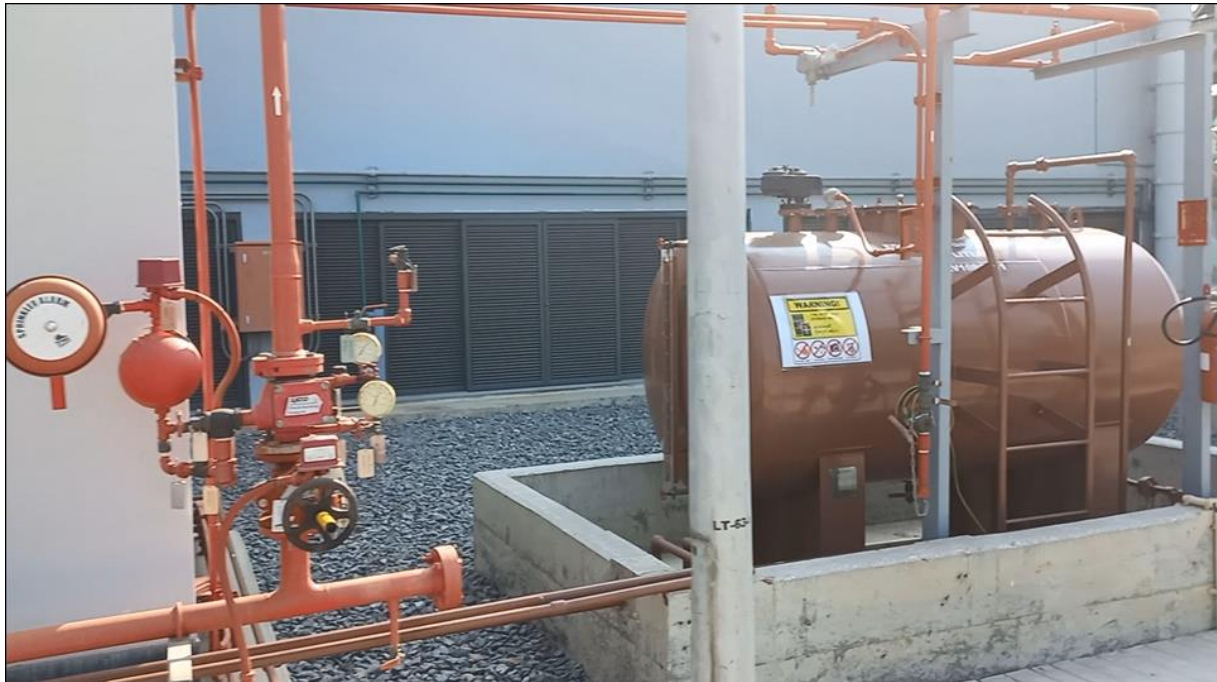
Photo 39: EDG Diesel Day Tank (Photo taken from video provided for January 2023 Site Visit)
