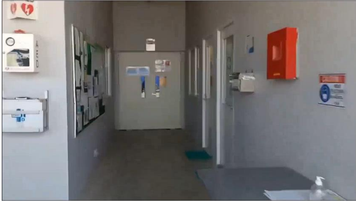
Photo 19: Entrance to the Warehouse ahead and Clinic on the right with AED Defibrillator and First Aid Kit on the left (Photo taken from video shared during January 2023 Site Visit)
