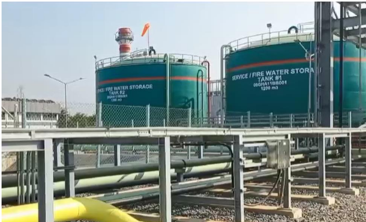
Photo 20: Two (2) fire water storage tanks of 1200 m 3 capacity each (Photo taken from video provided for January 2023 Site Visit)
