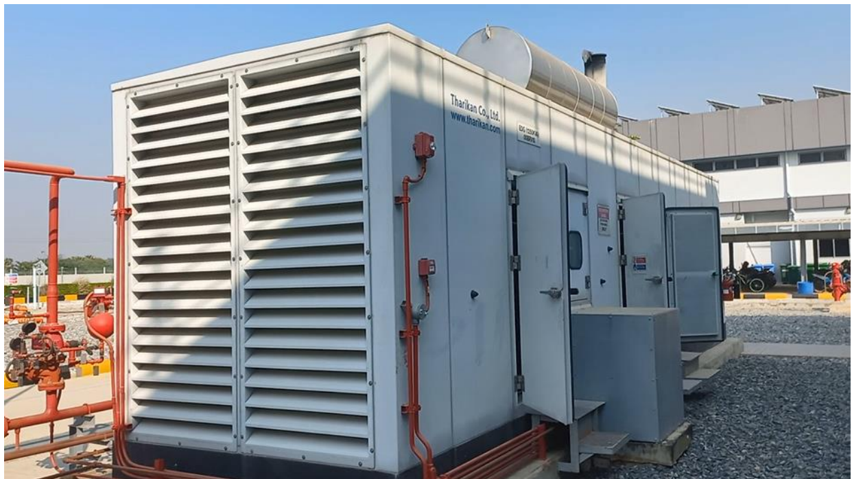
Photo 40: Diesel Generator/EDG Genset (Photo taken from video provided for January 2023 Site Visit)
