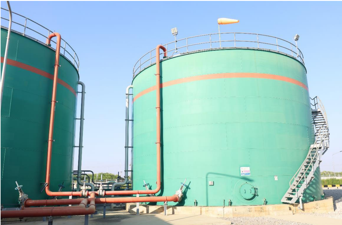
Photo 8: Water Storage Tanks next to Central Monitoring Basin (Photo taken from video provided during January 2025 Site Visit)
