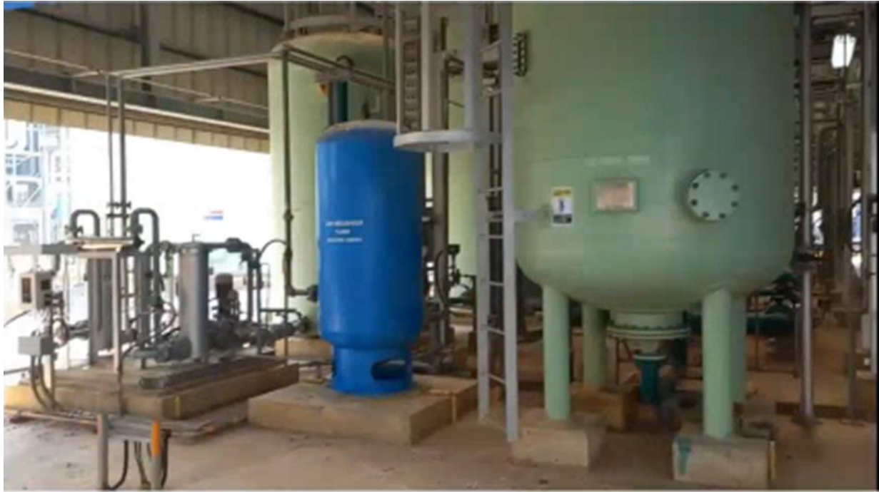
Photo 31: Water treatment plant (Photo taken from video shared during January 2023 Site Visit)
