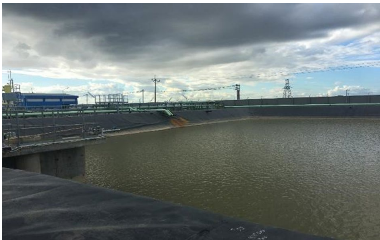
Photo 6: River water storage reservoir
