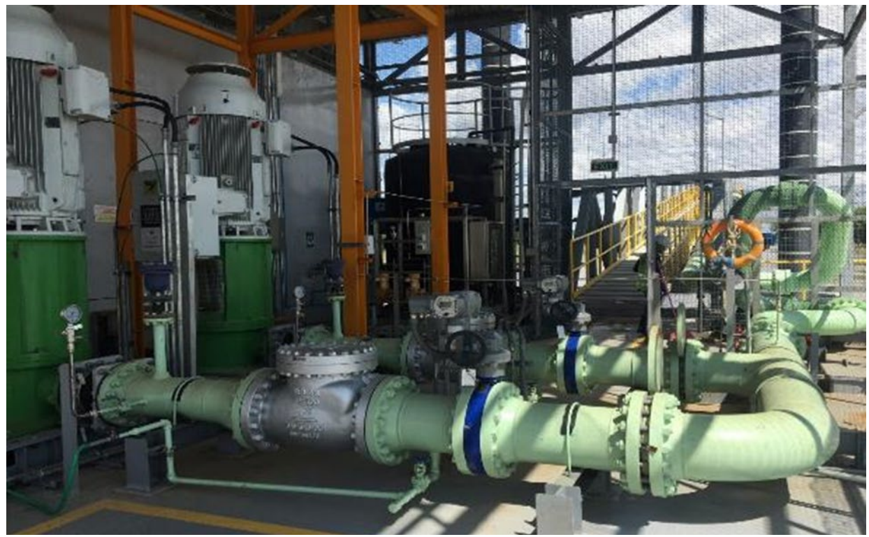
Photo 16: River water supply pumps
