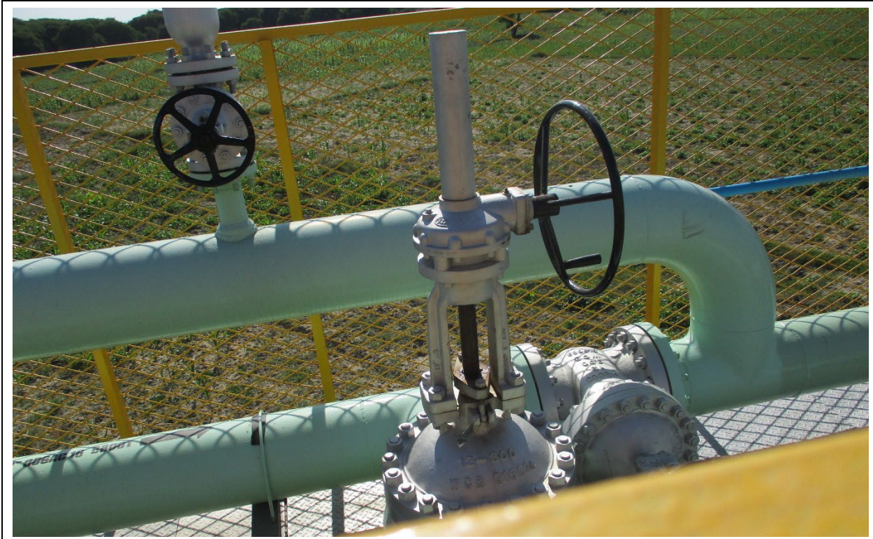
Photo 18: Plant designated quarterly water sampling location from the discharge pipeline
