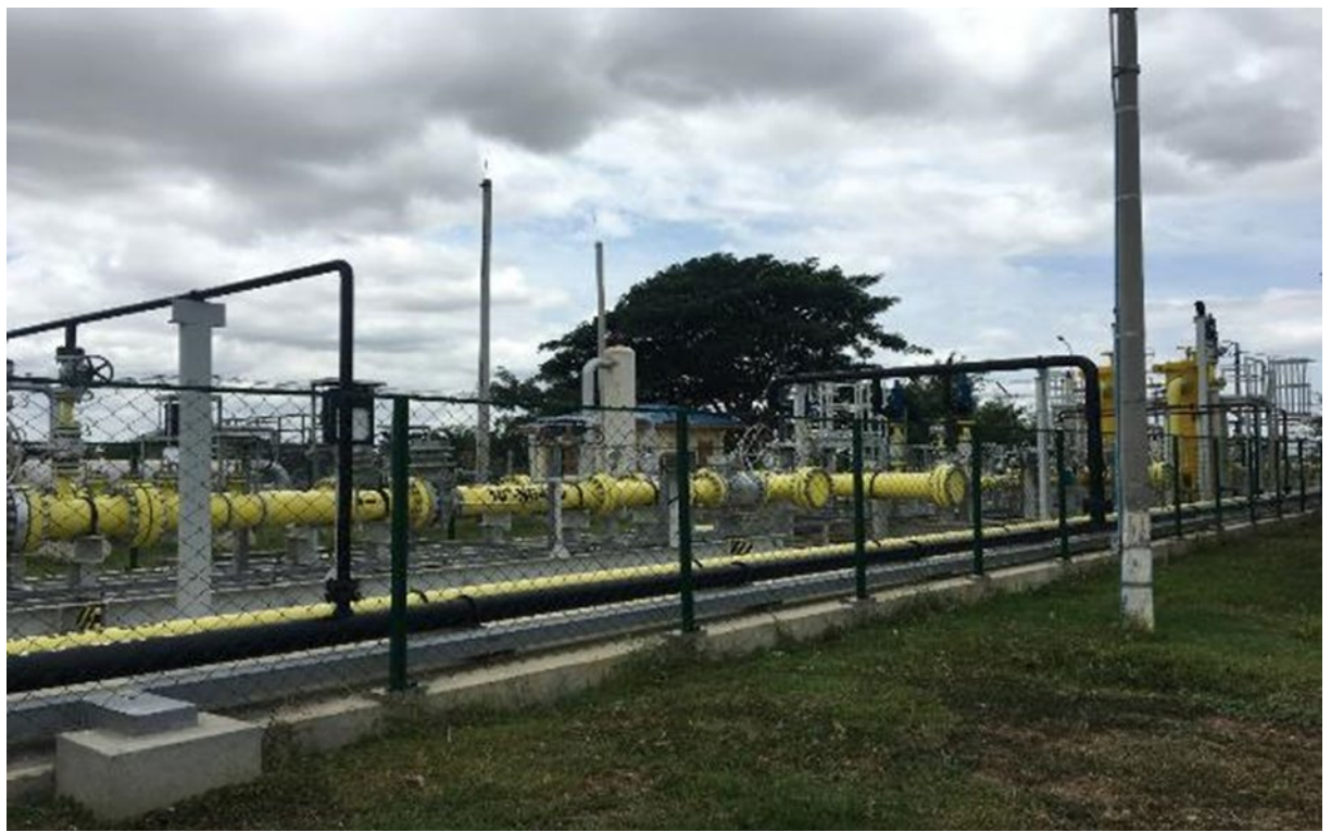
Photo 12: MOGE gas receiving station
