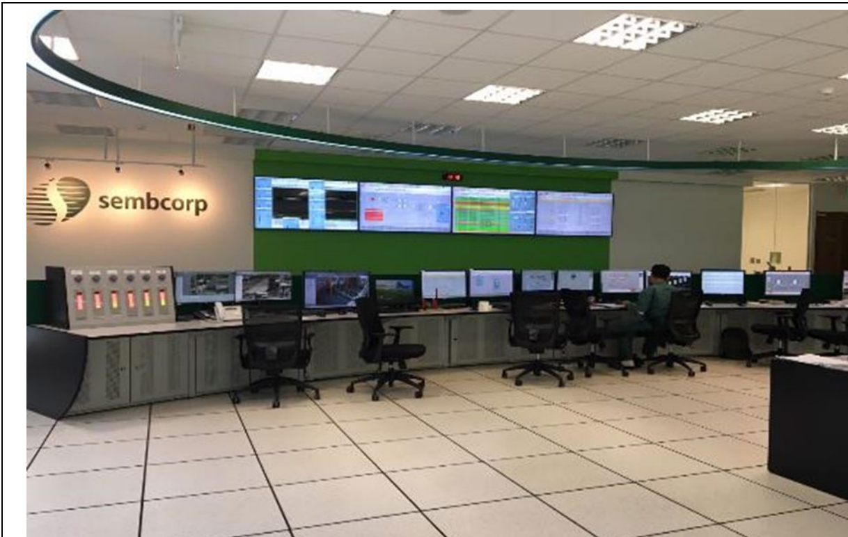
Photo 3: Plant Control Room with Continuous Operations Monitoring System within the main administration building
