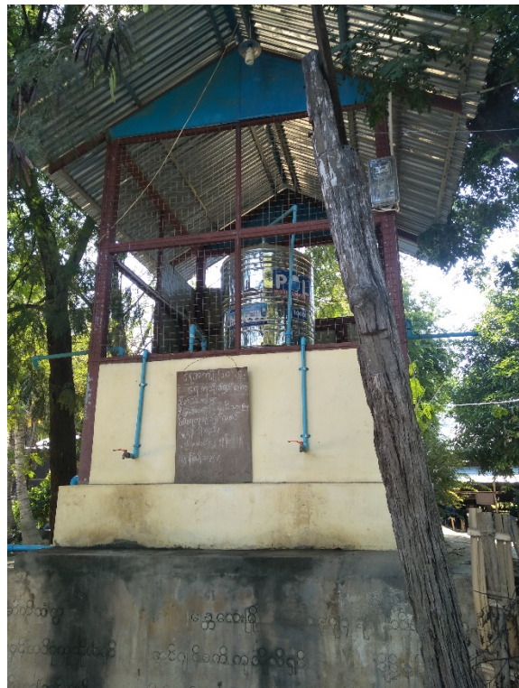
Photo 26: Water Treatment Plant, Seik Nyan Village
