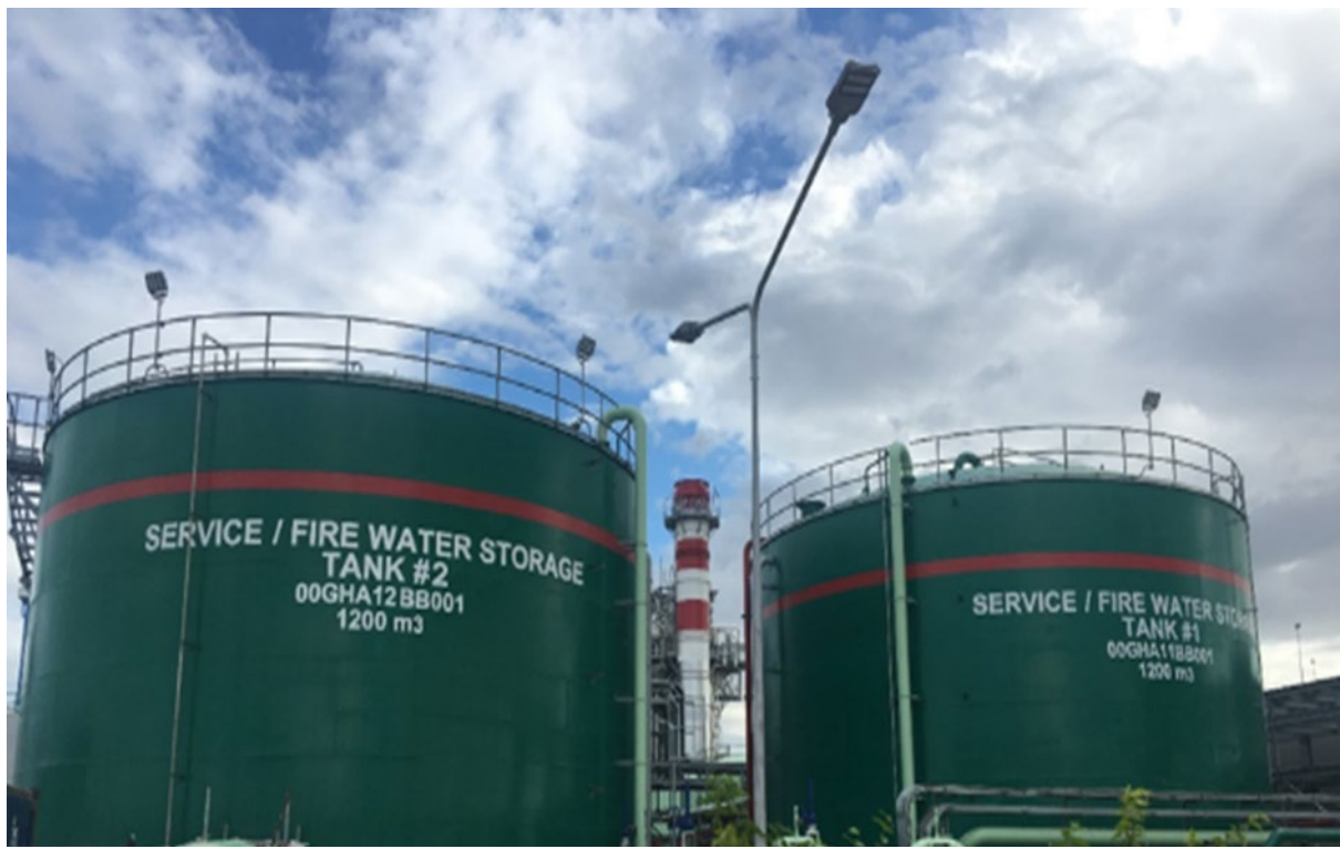
Photo 9: Two (2) fire water storage tanks of 1200 m 3 capacity each
