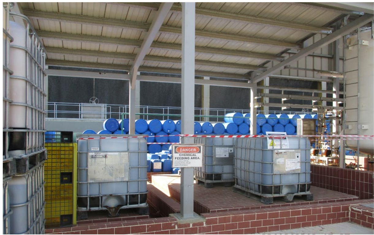
Photo 10: Chemical feeding area is roofed and contained within a bunded area.
