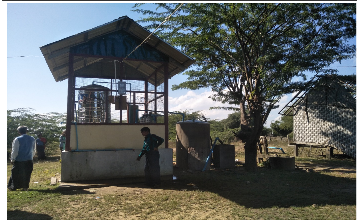
Photo 23: Water Treatment Plant, Tha Pyay Thar Village
