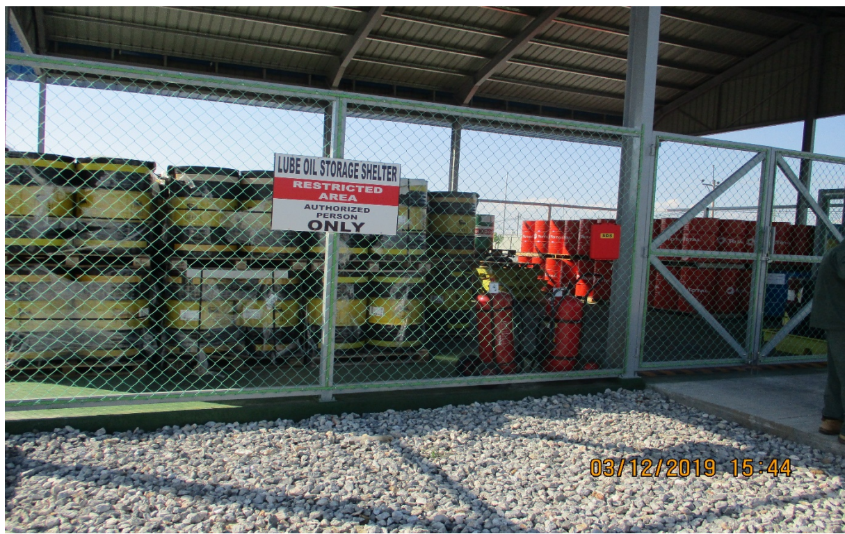
Photo 8: The lubricant oil storage area is paved, roofed and access controlled.
