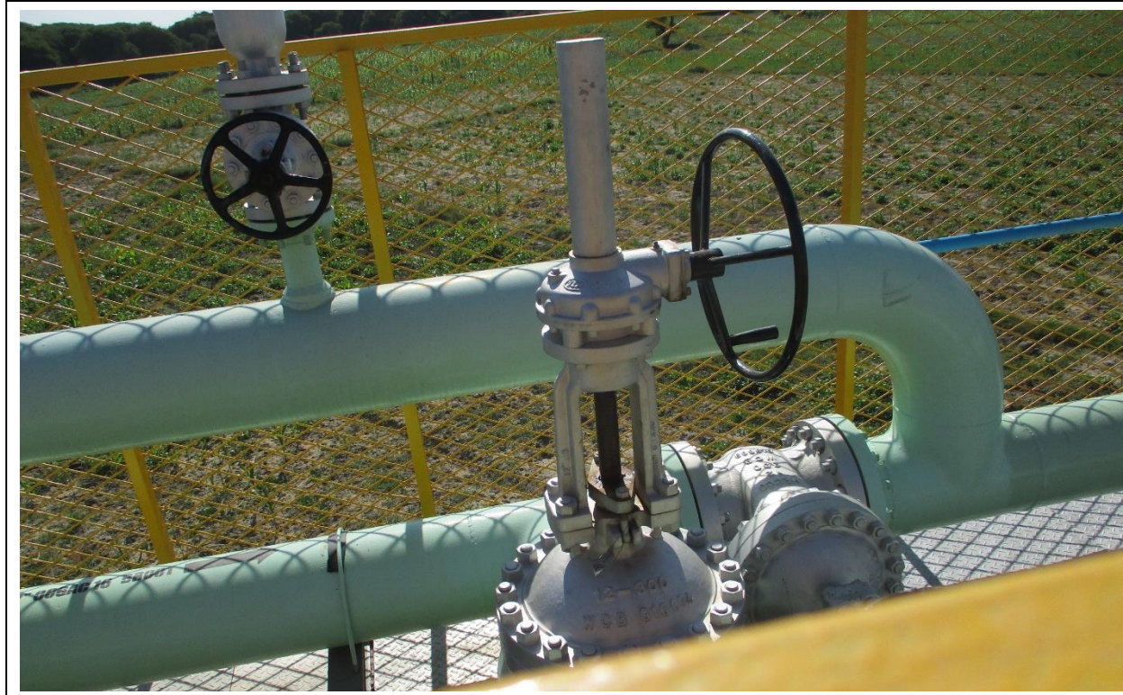
Photo 17: Designated water sampling location from the discharge pipeline (December 2019)
