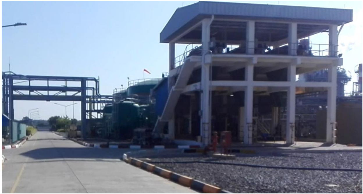
Photo 3: Views of the plant exterior (Photo taken from live video during December 2020 Audit)
