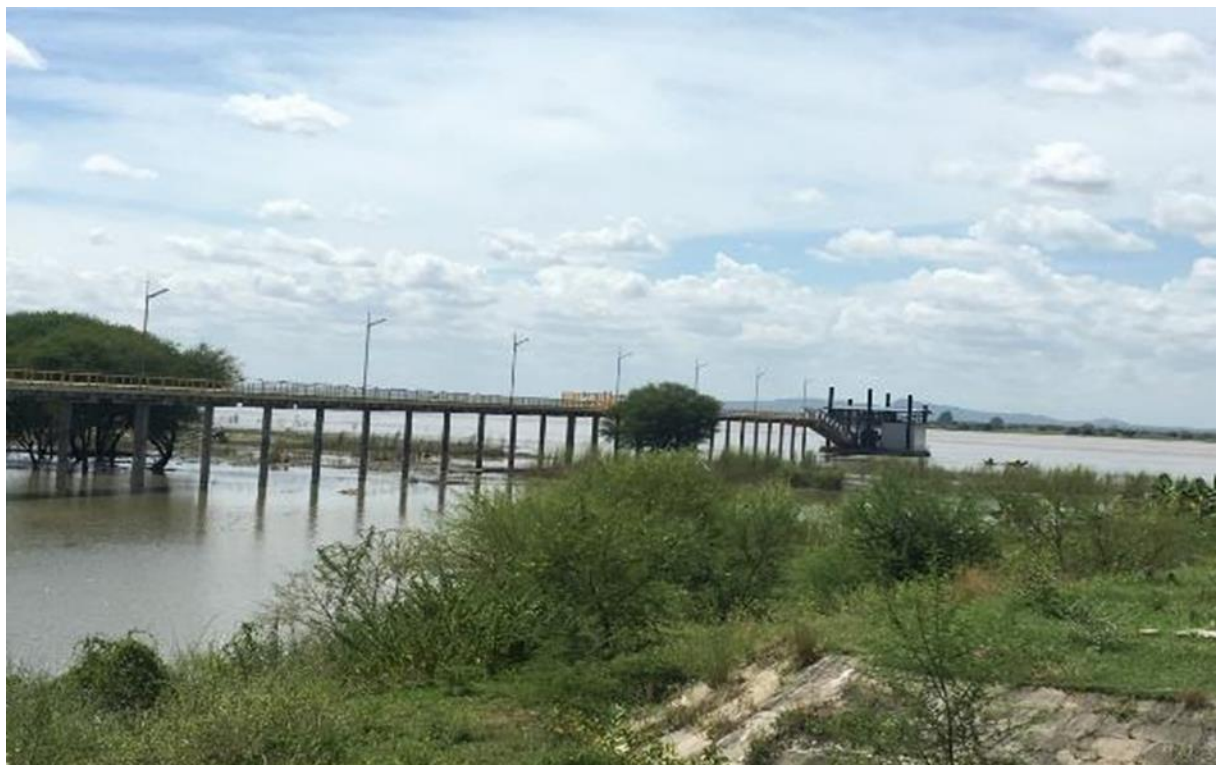
Photo 15: Overview of the river water supply pipeline and pumping station (December 2019)
