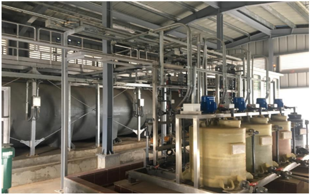
Photo 11: Sanitary wastewater treatment plant (December 2019)
