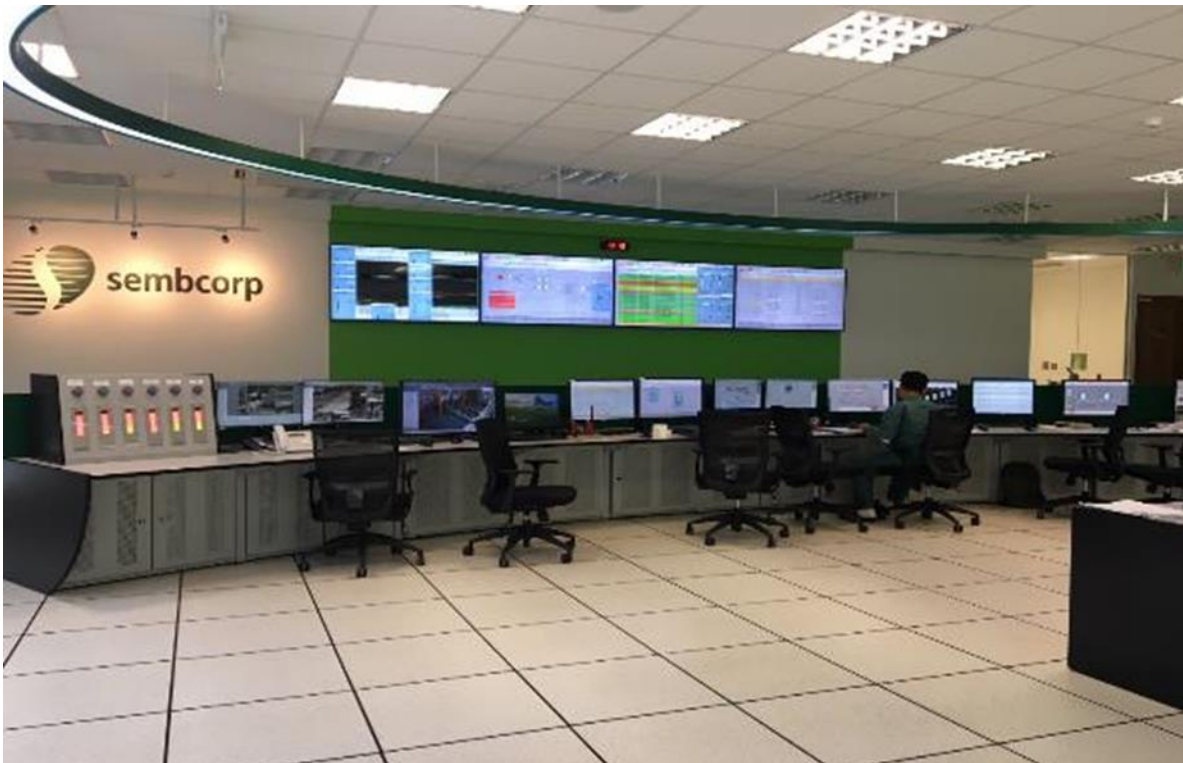
Photo 3: Plant Control Room with Continuous Operations Monitoring System within the main Administration Building (December 2019)
