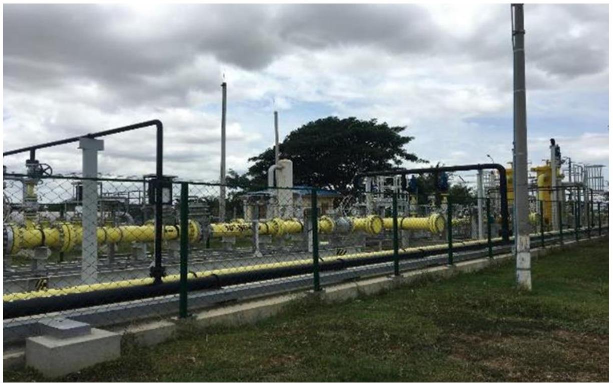
Photo 12: MOGE gas receiving station (December 2019)
