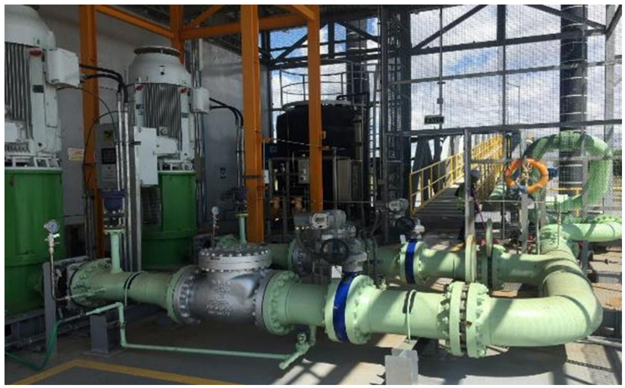
Photo 16: River water supply pumps (December 2019)
