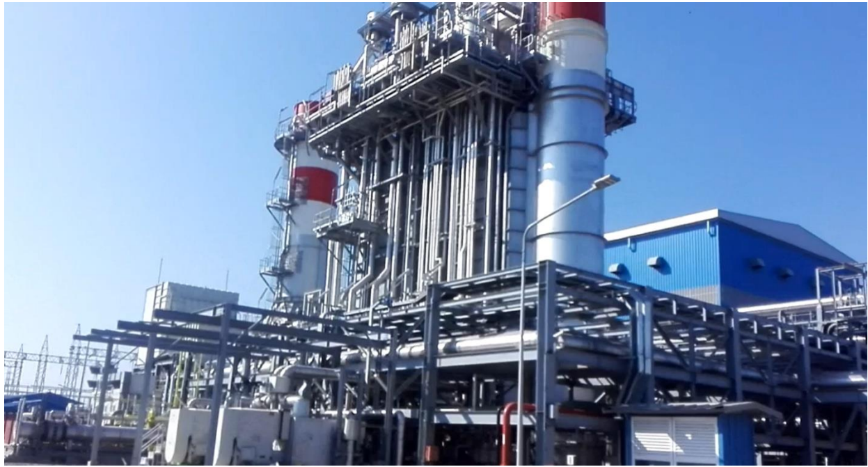
Photo 1: View of the Myingyan CCGT Plant (Photo taken from live video during December 2020 Audit)
