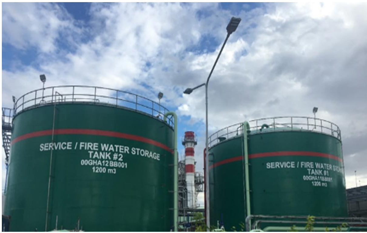
Photo 9: Two (2) fire water storage tanks of 1200 m 3 capacity each (December 2019)
