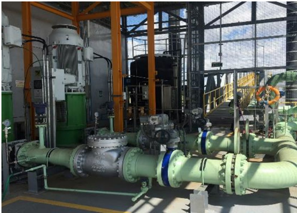
Photo 4: River water supply pumps (December 2019)
