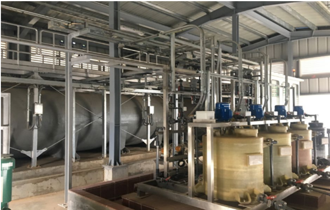
Photo 2: Sanitary wastewater treatment plant (December 2019)
