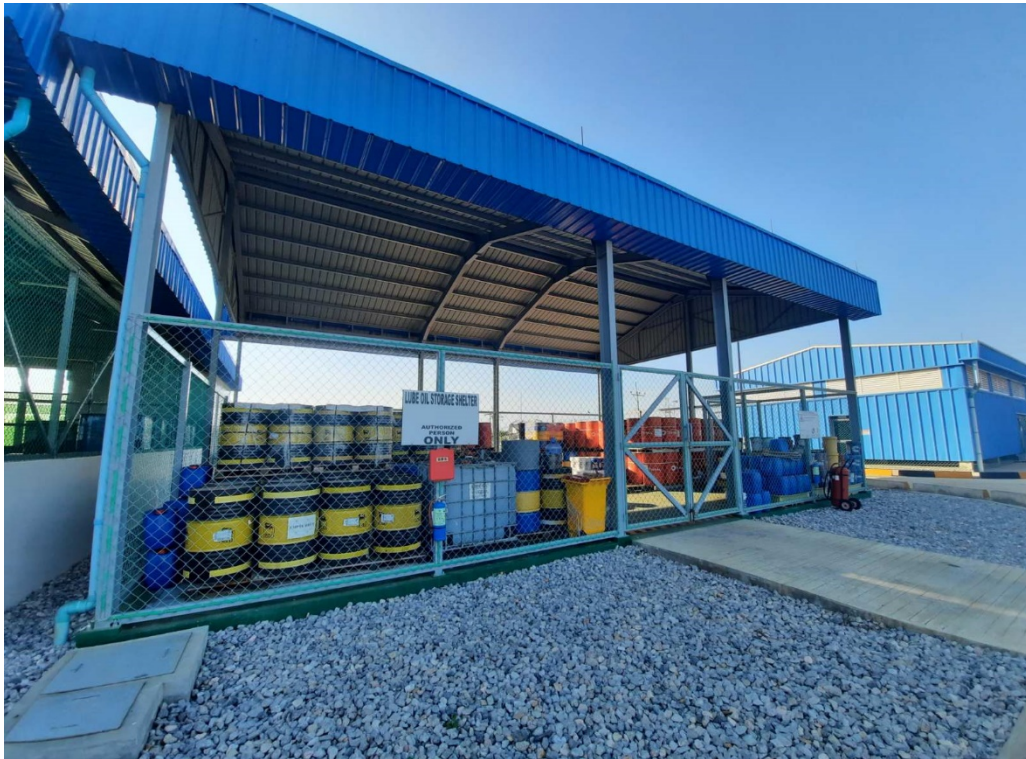
Photo 14: Used oil stored at Lub Oil Shelter (Photo provided by SMPC, January 2021)
