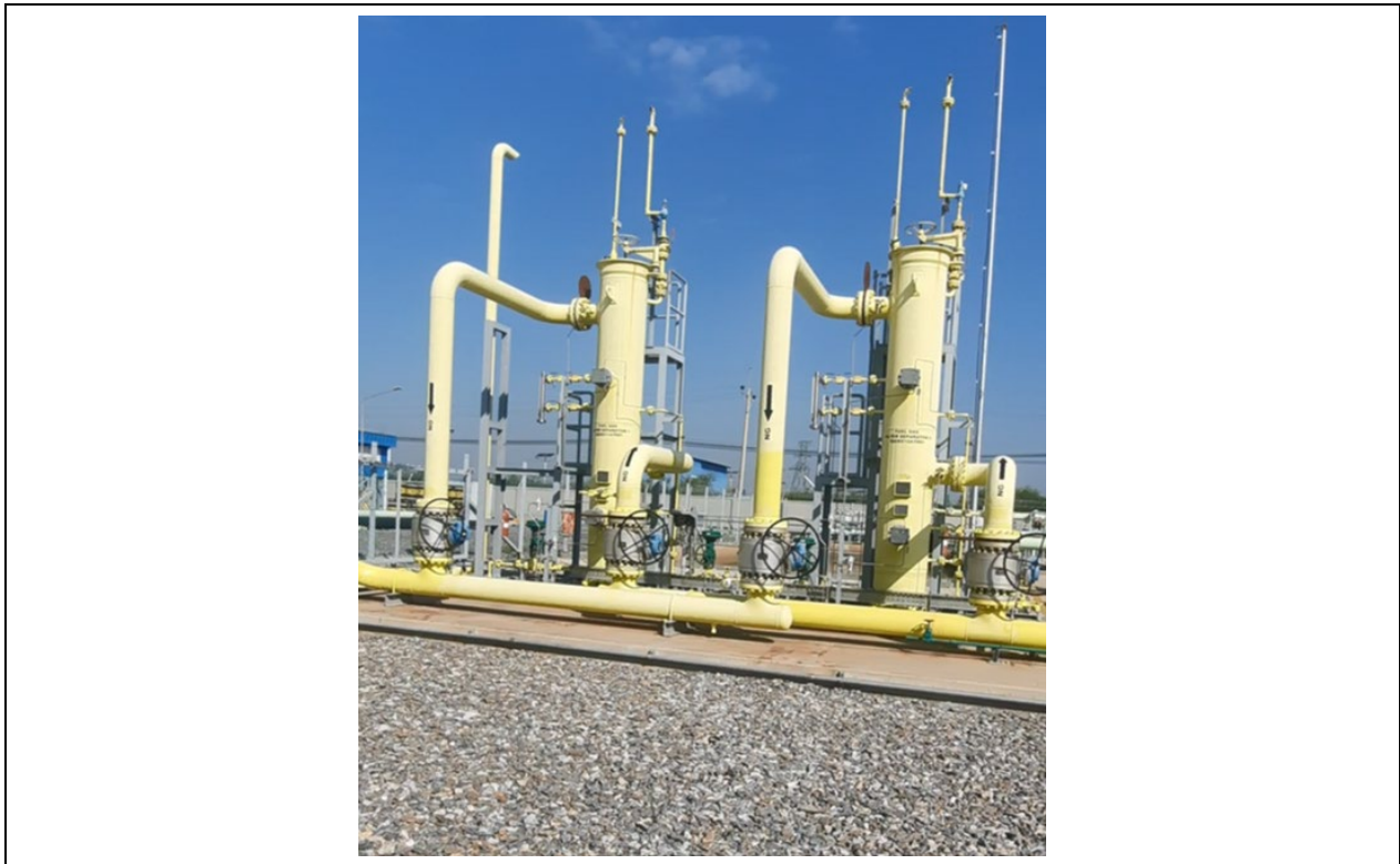
Photo 18: MOGE gas receiving station (Photo taken from video provided by SMPC, January 2022)
