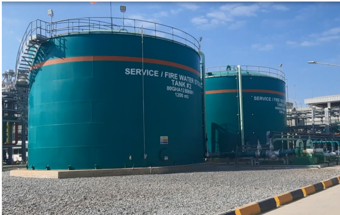
Photo 15: Two (2) fire water storage tanks of 1200 m 3 capacity each (Photo taken from live video during February 2022 Audit)
