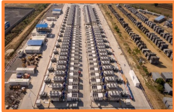
V Power 90 MW
