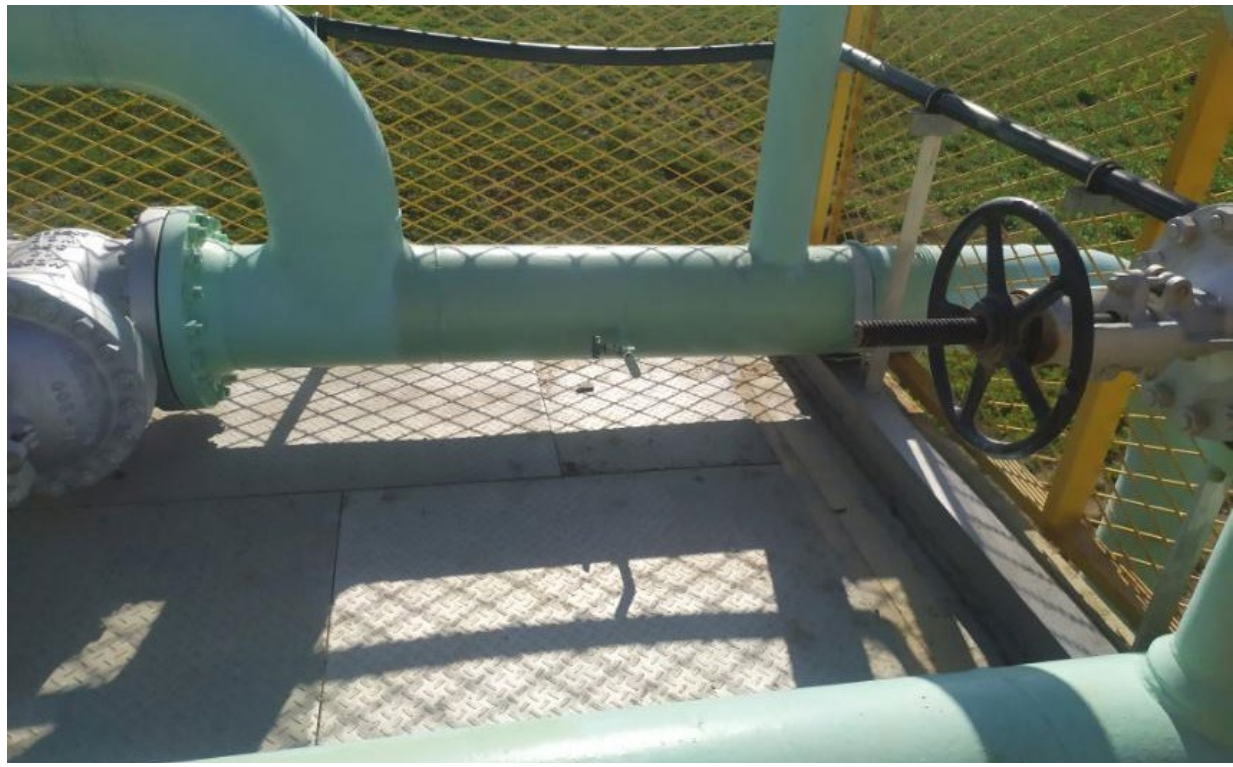
Photo 23: Designated water sampling location from the discharge pipeline (Photo provided by SMPC, January 2022)
