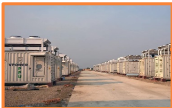
V Power 133 MW
