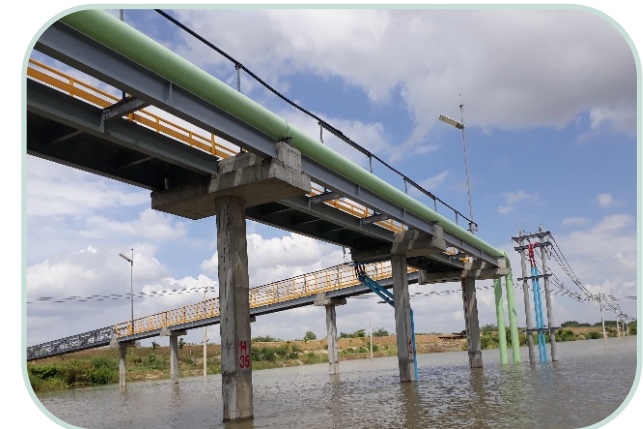
Water Pipeline (Intake & Discharge)
