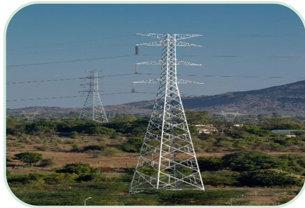
230 kV Transmission Tower
