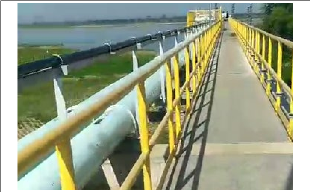
Photo 21: Bridge access and river water supply pipeline leading to pumping station (Photo taken from video provided by SMPC, January 2022)
