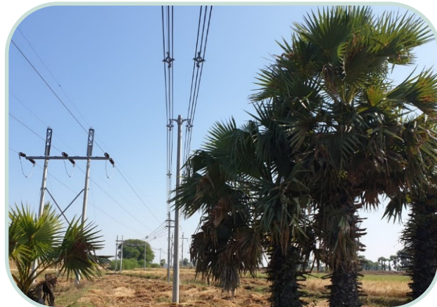
6.6kV Overhead Transmission Line
