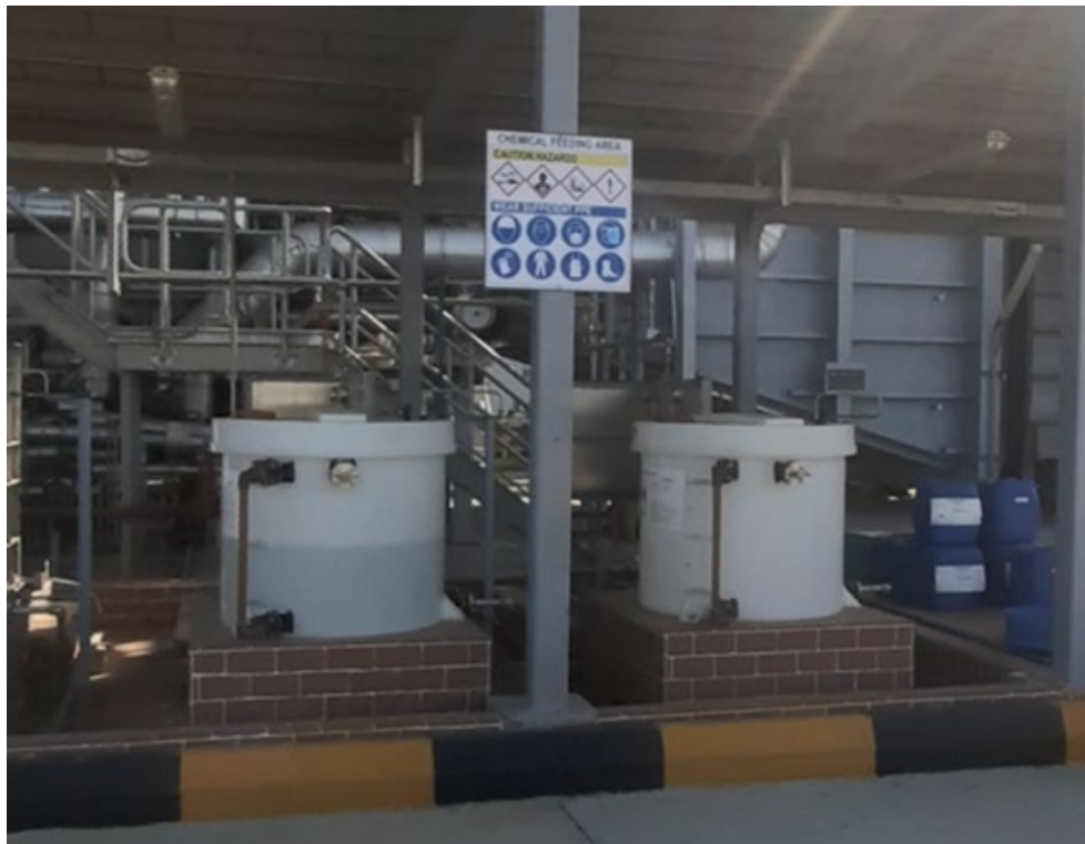
Photo 16: Chemical feeding area (Photo taken from video provided by SMPC, January 2022)
