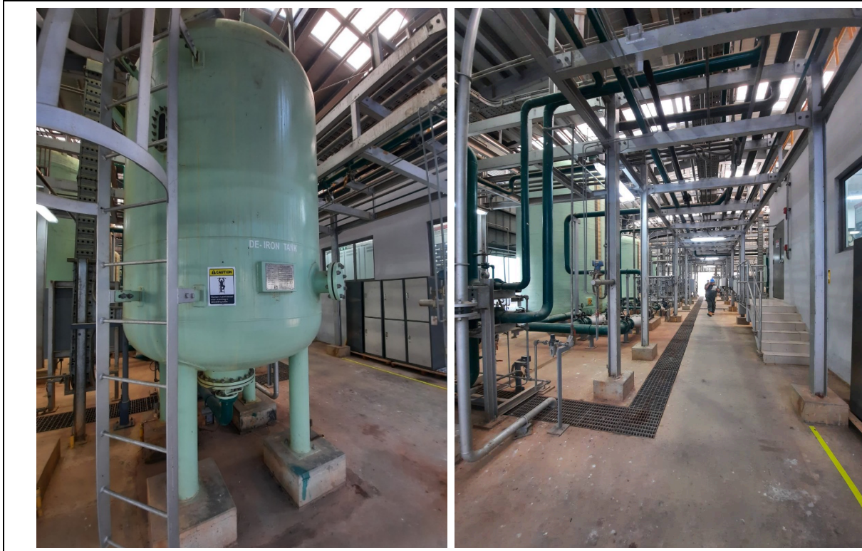
Photo 17: Water treatment plant (Photo provided by SMPC, January 2022)
