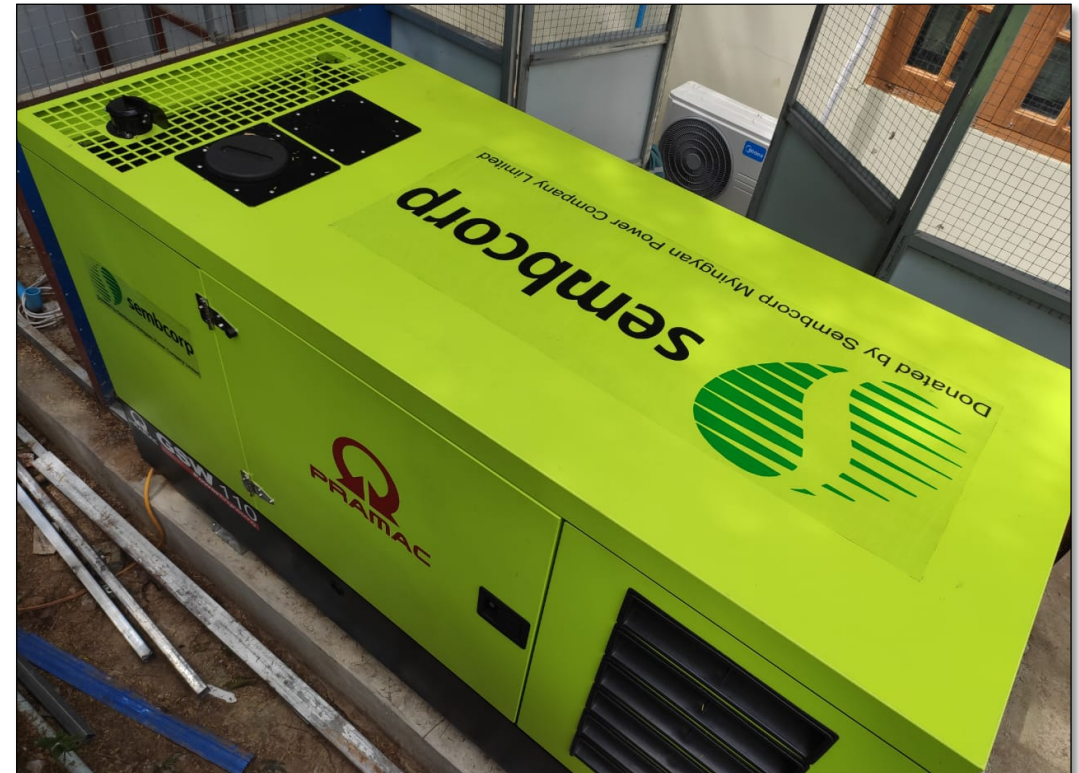
Supported 100kVA generator to Myingyan District Hospital purpose to use COVID-19 treatments as well as others medical usage in hospital
