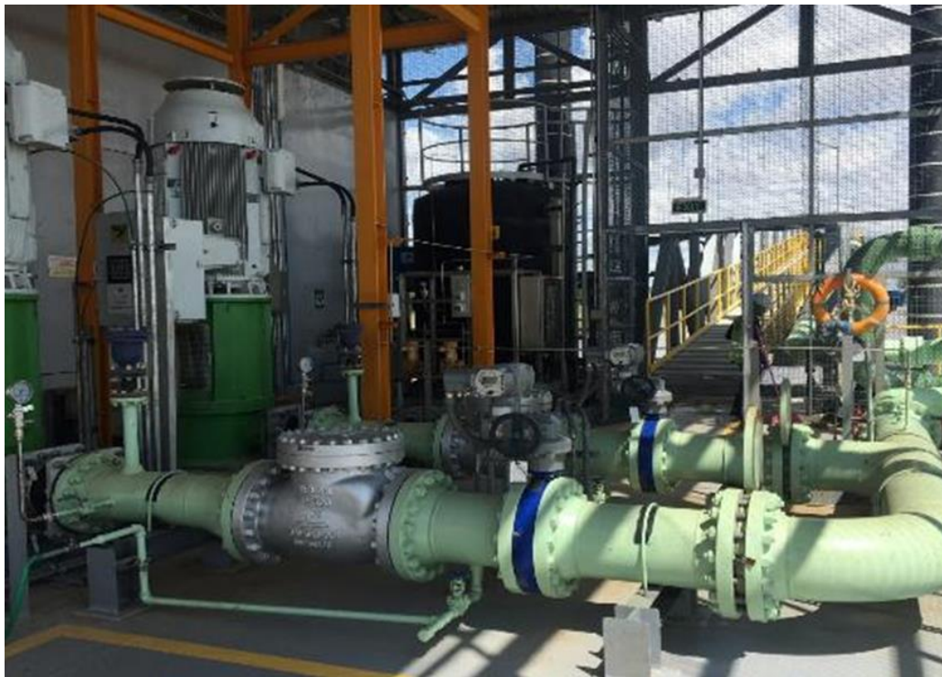
Photo 4: River water supply pumps (December 2019)
