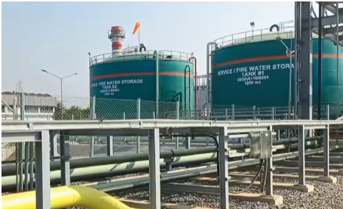
Photo 6: Two (2) fire water storage tanks of 1200 m 3 capacity each (Photo taken from video provided for January 2023 audit)
