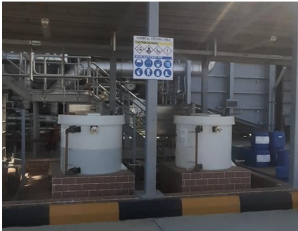
Photo 7: Chemical feeding area (Photo taken from video provided by SMPC, January 2022)
