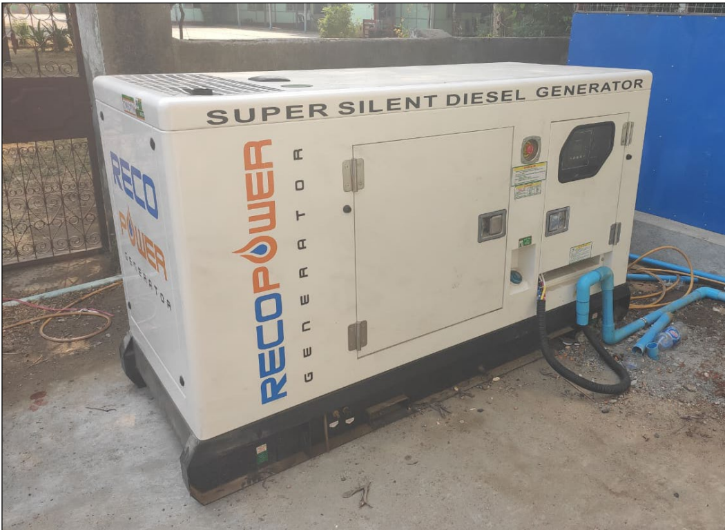
Supported 30kVA generator to Myingyan District Hospital purpose to use COVID-19 treatments as well as others medical usage in hospital
