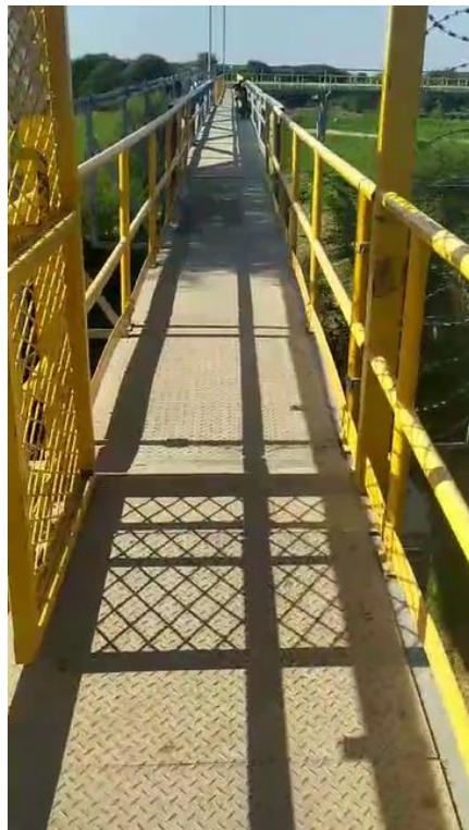
Photo 8: Entrance leading to the river water supply pumping station (Photo taken from video provided by SMPC, January 2022)
