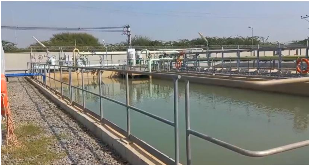
Photo 8: Central Monitoring Basin of water storage reservoir (Photo taken from video shared during January 2023 audit)
