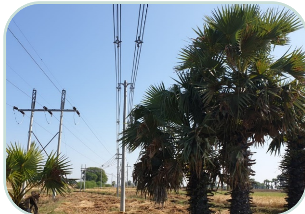
6.6kV Overhead Transmission Line
