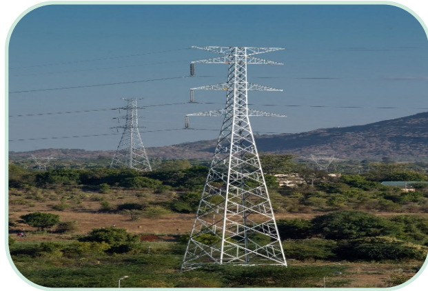
230 kV Transmission Tower
