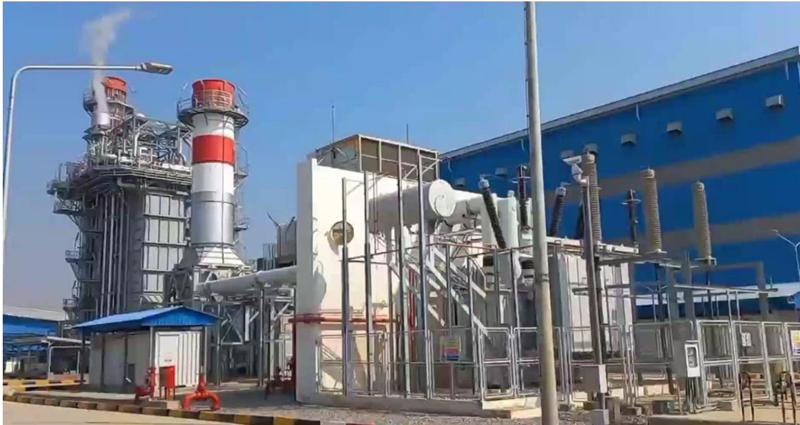
Photo 4: View of Unit 1 plant exterior (Photo taken from video shared during January 2023 audit)
