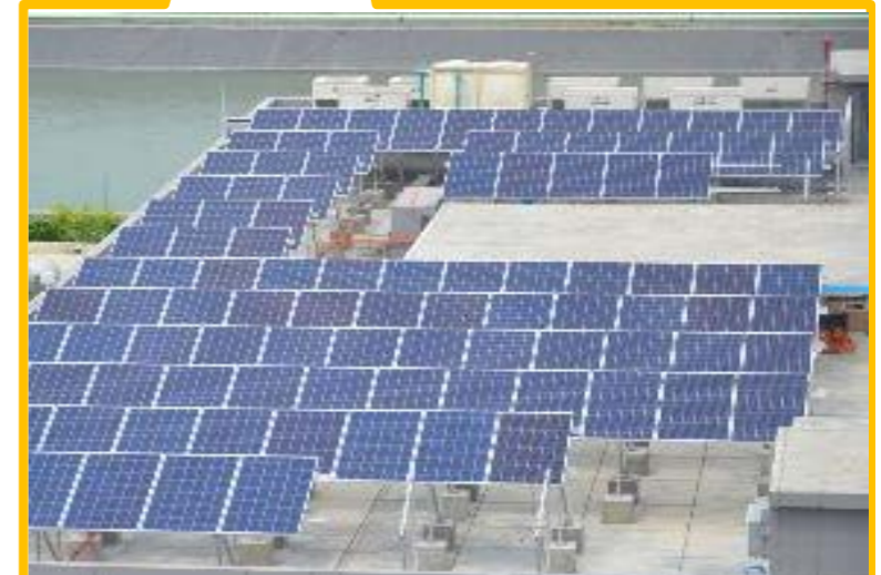
Solar Panel in Admin Building
