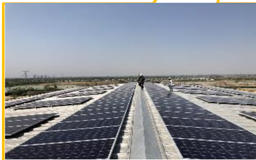
Solar Panel in Warehouse
