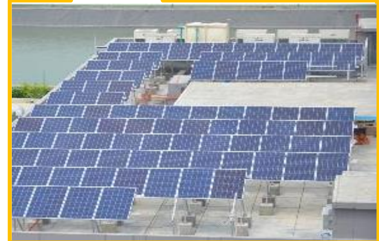
Solar Panel in Admin Building
