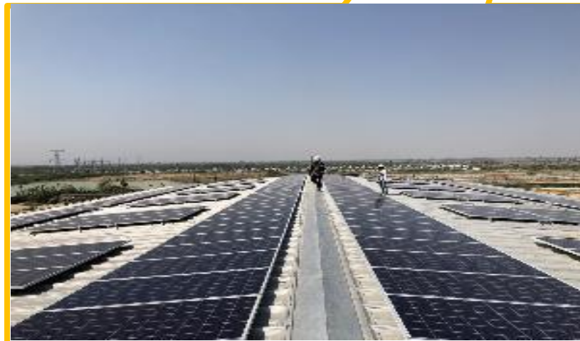
Solar Panel in Warehouse
